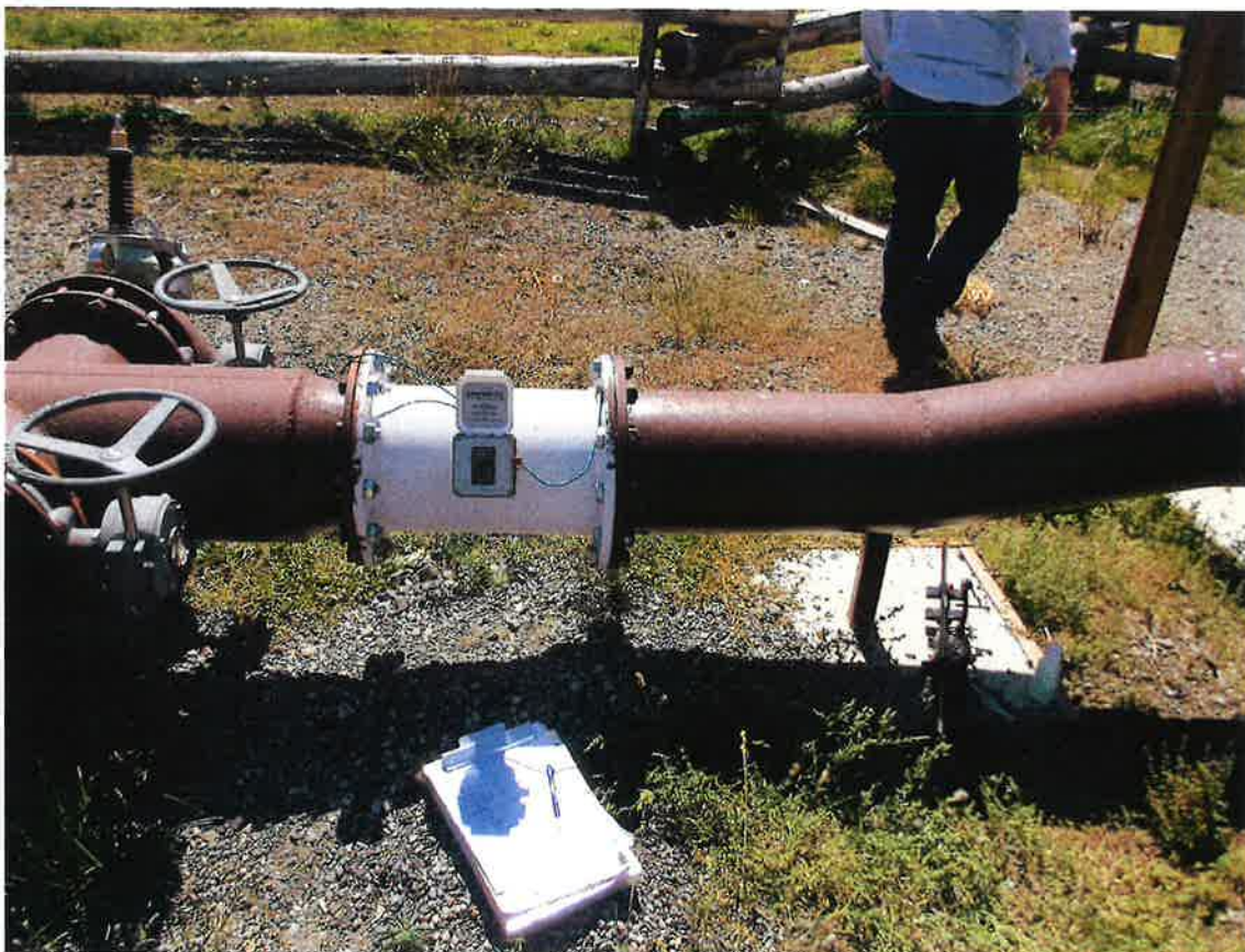
Meter installation at upper well
