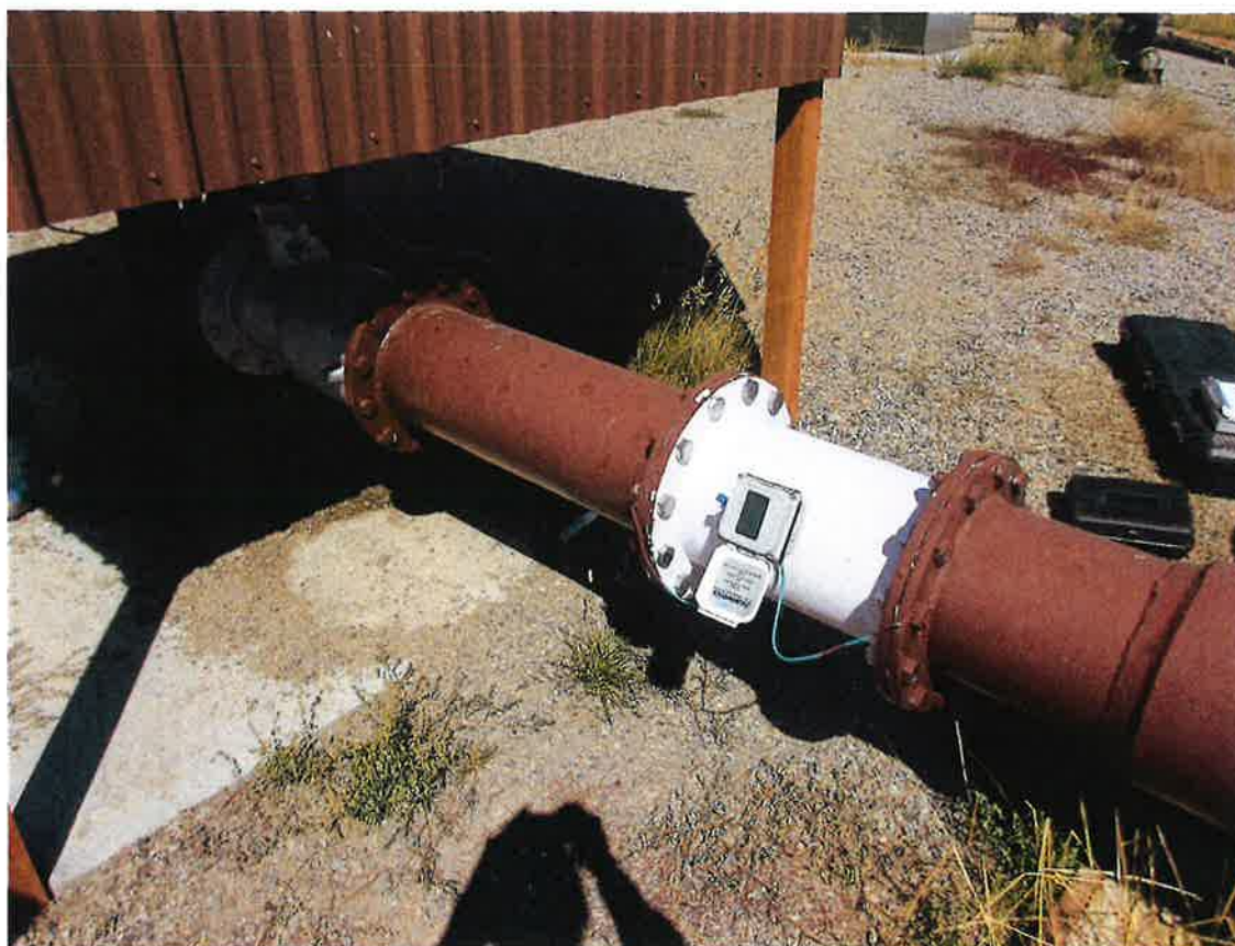
Meter installation at lower well
