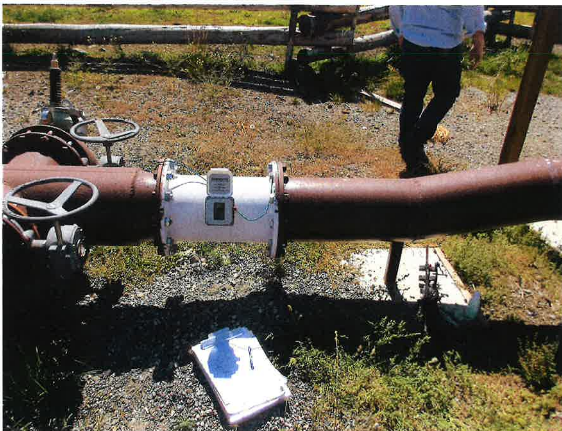
Meter installation at upper well
