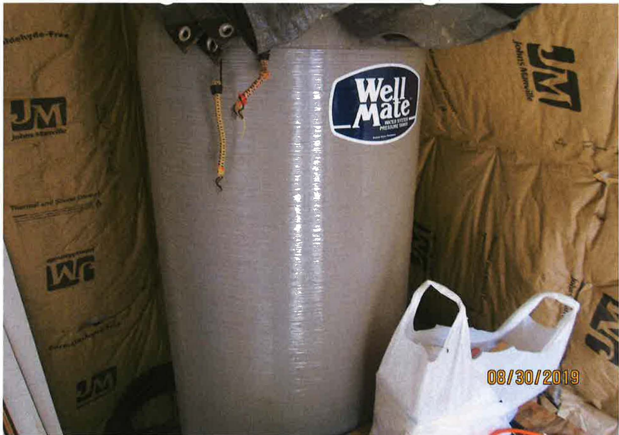
Water is diverted to pressure tank. Unable to perform flow measurement due to inadequate space.
