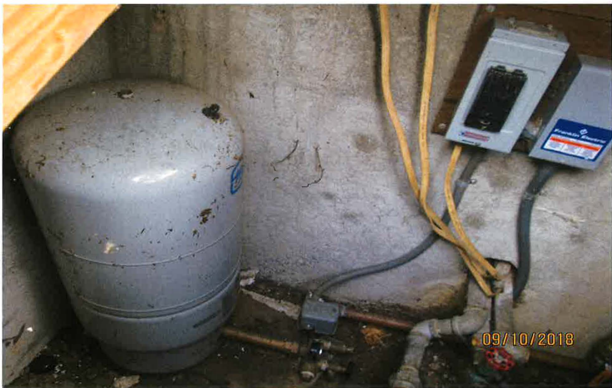
Water diverted from lake directly into pressure tank.
