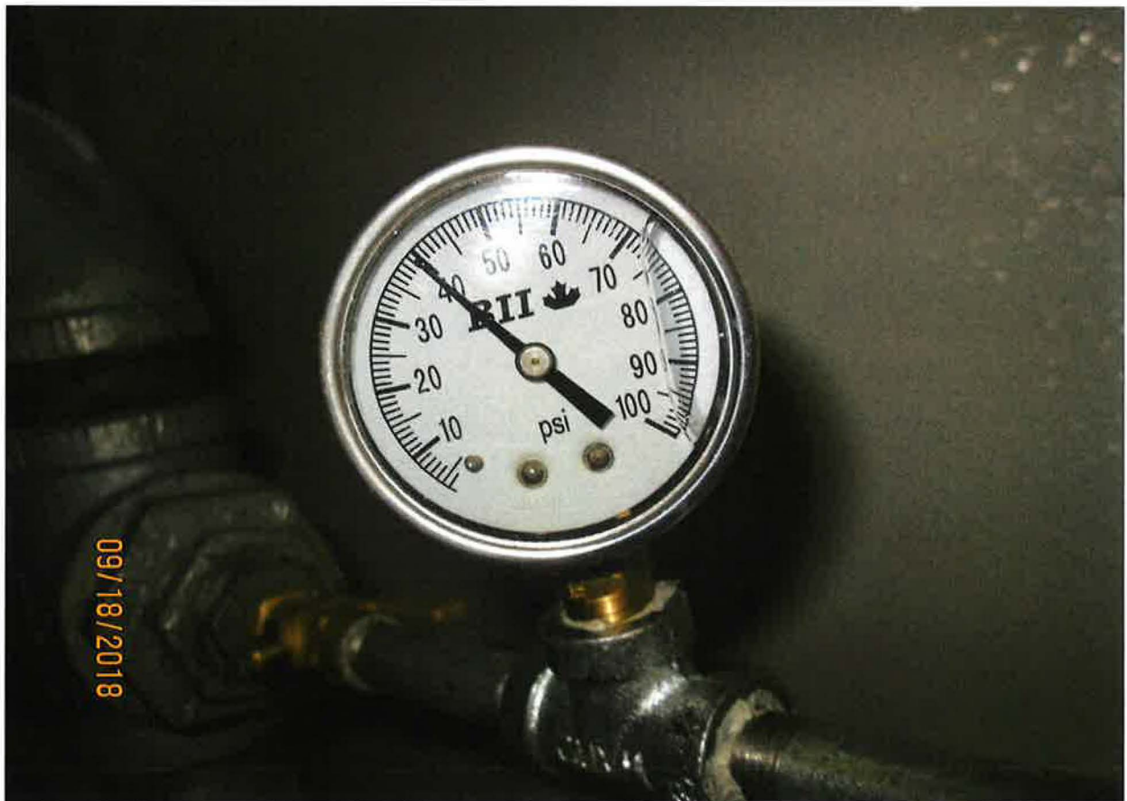
PUMP OPERATING PRESSURE 40 PSI
