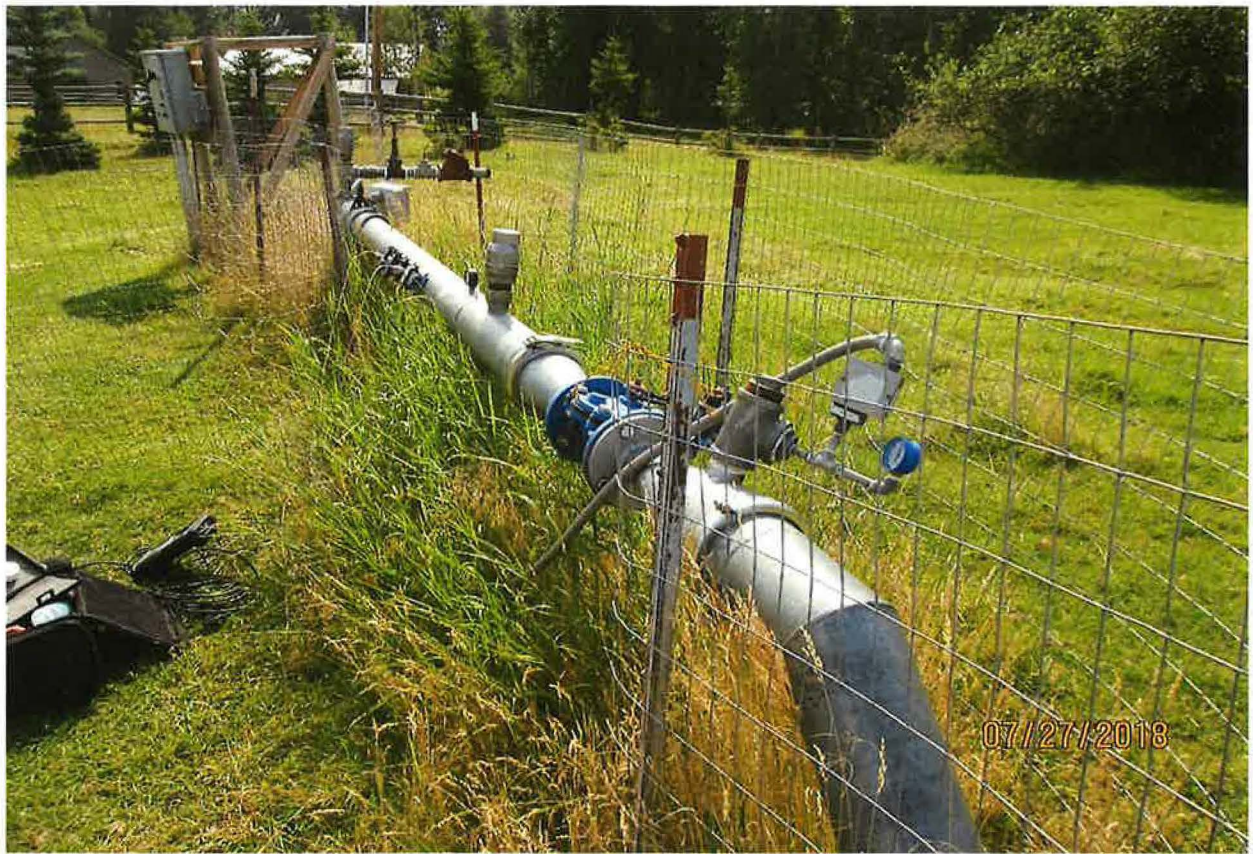
Section of pipe used for flow measurement.
