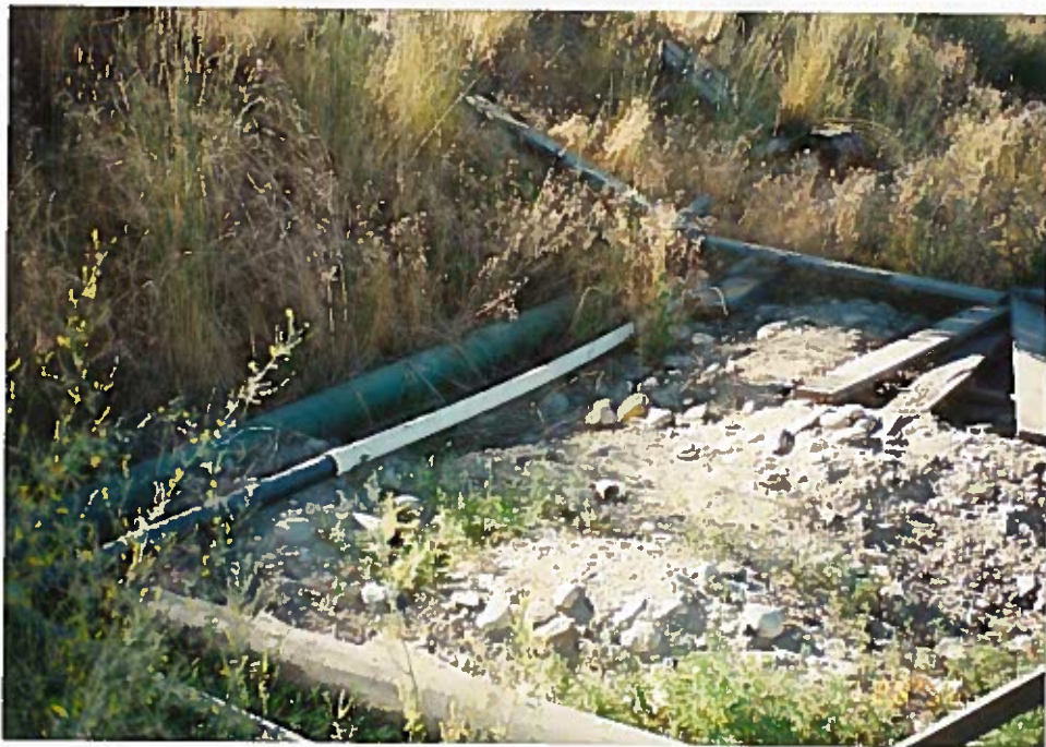
Discharge Pipe where measurement was taken
