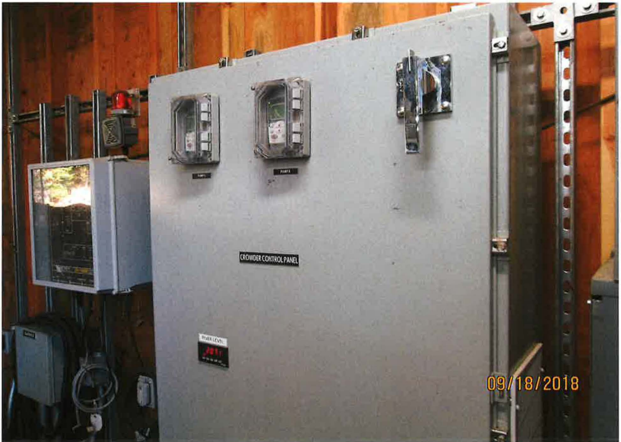
SYSTEM CONTROL PANEL
