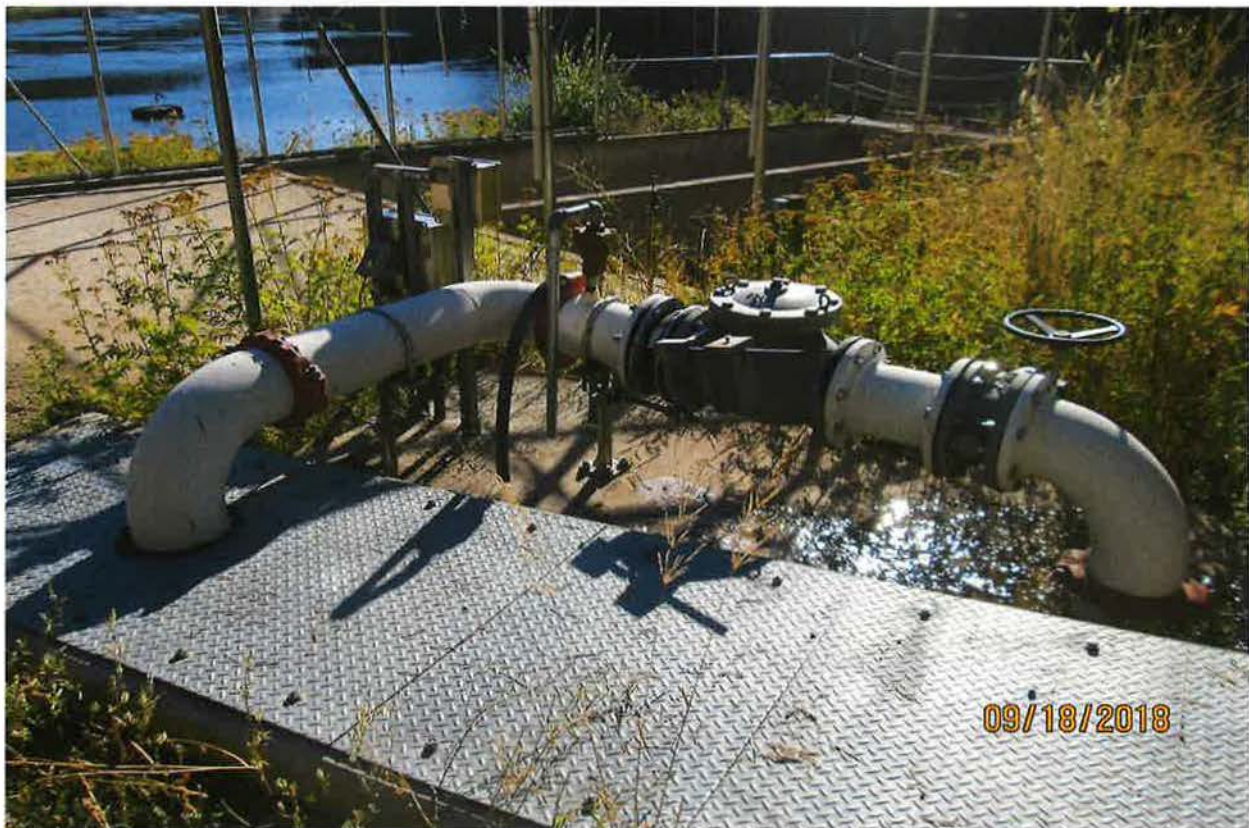
POD – 20 HP PUMP DIVERTS FROM RIVER
