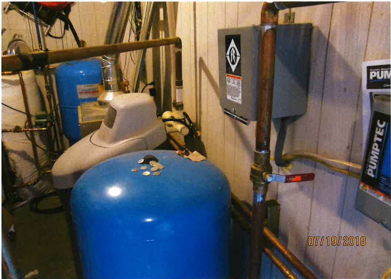
PRESSURE TANK / PUMP ROOM
