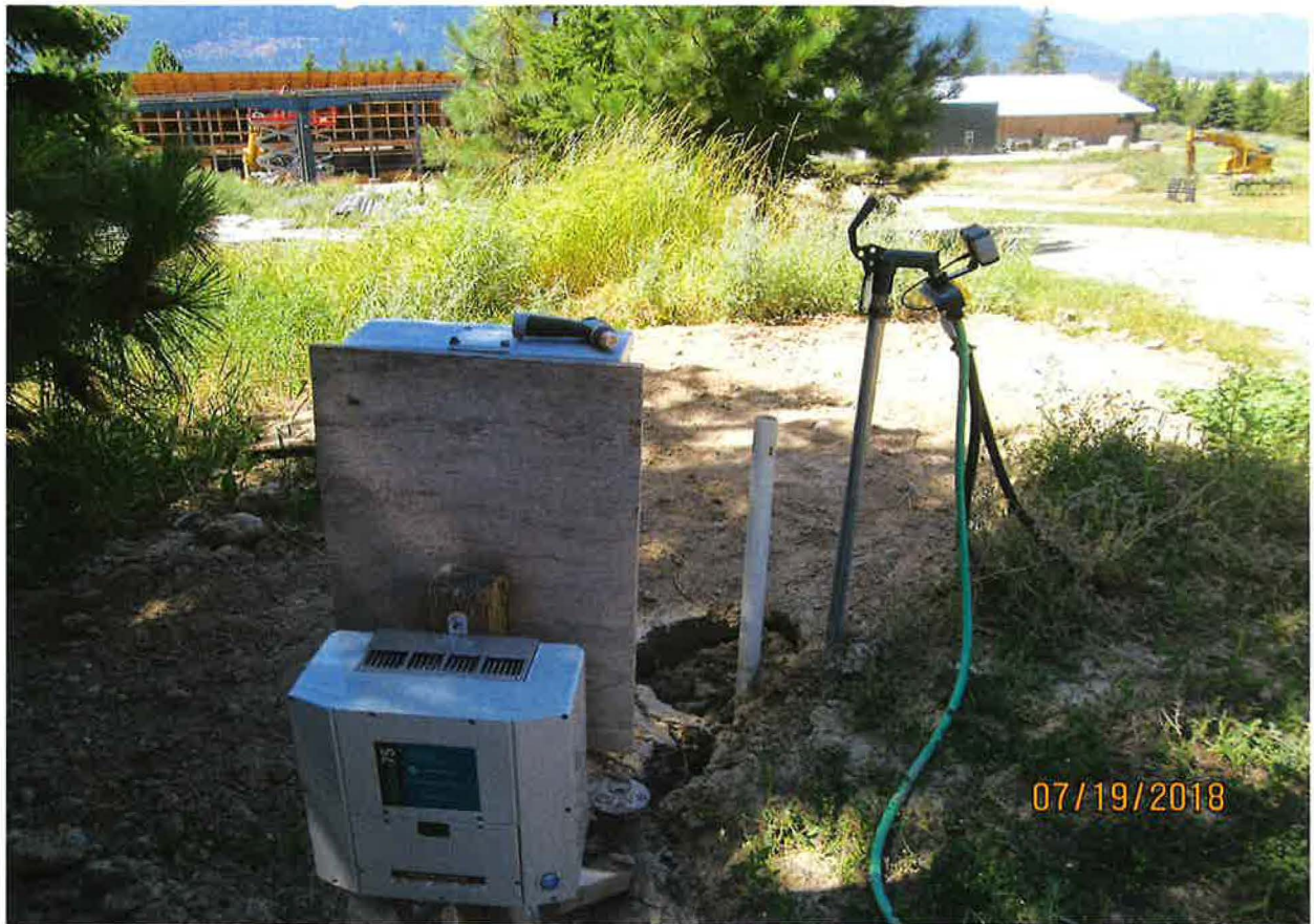
WELL AND ELECTRICAL SYSTEM
