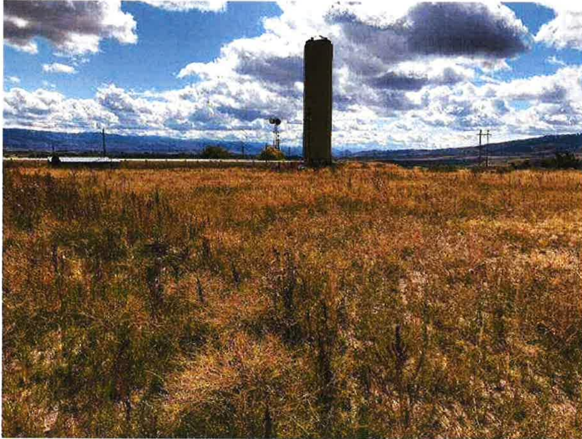
Upper Cathodic Protection Ground Bed with Surge Tower in Distance, Viewing Southwest
