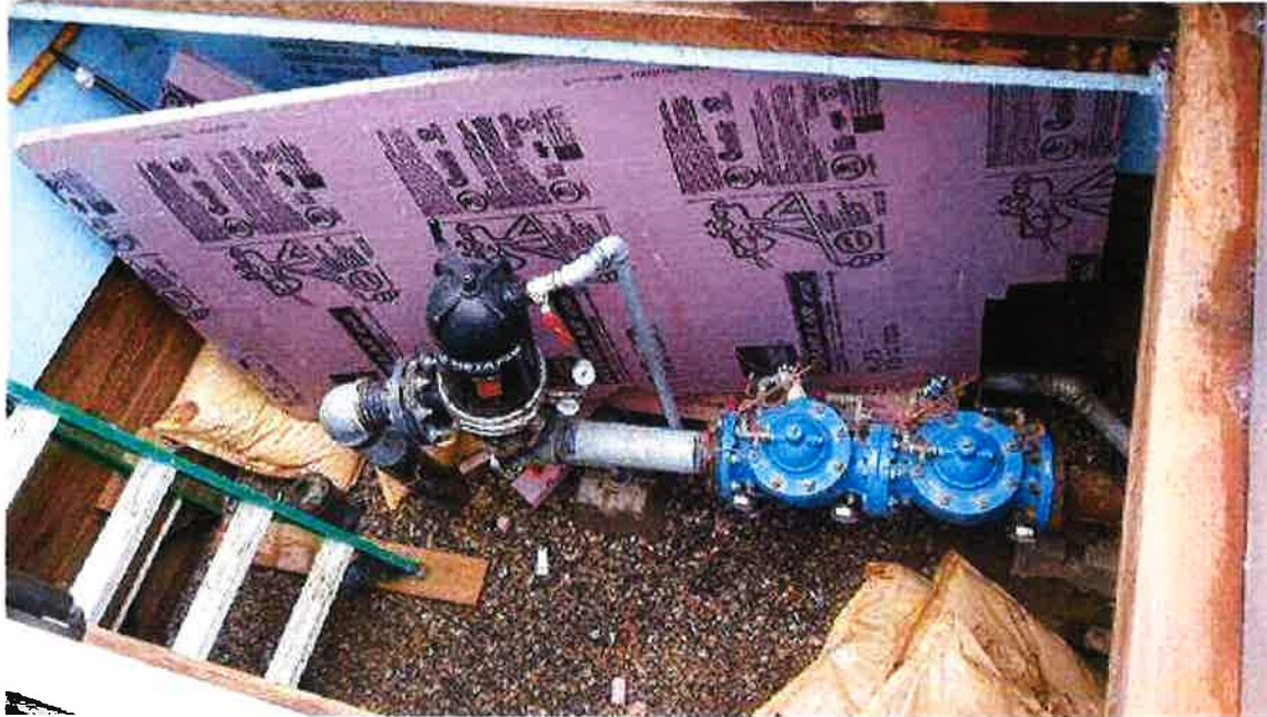
Inside Lower Ground Bed Penstock Tap/Valve Box
