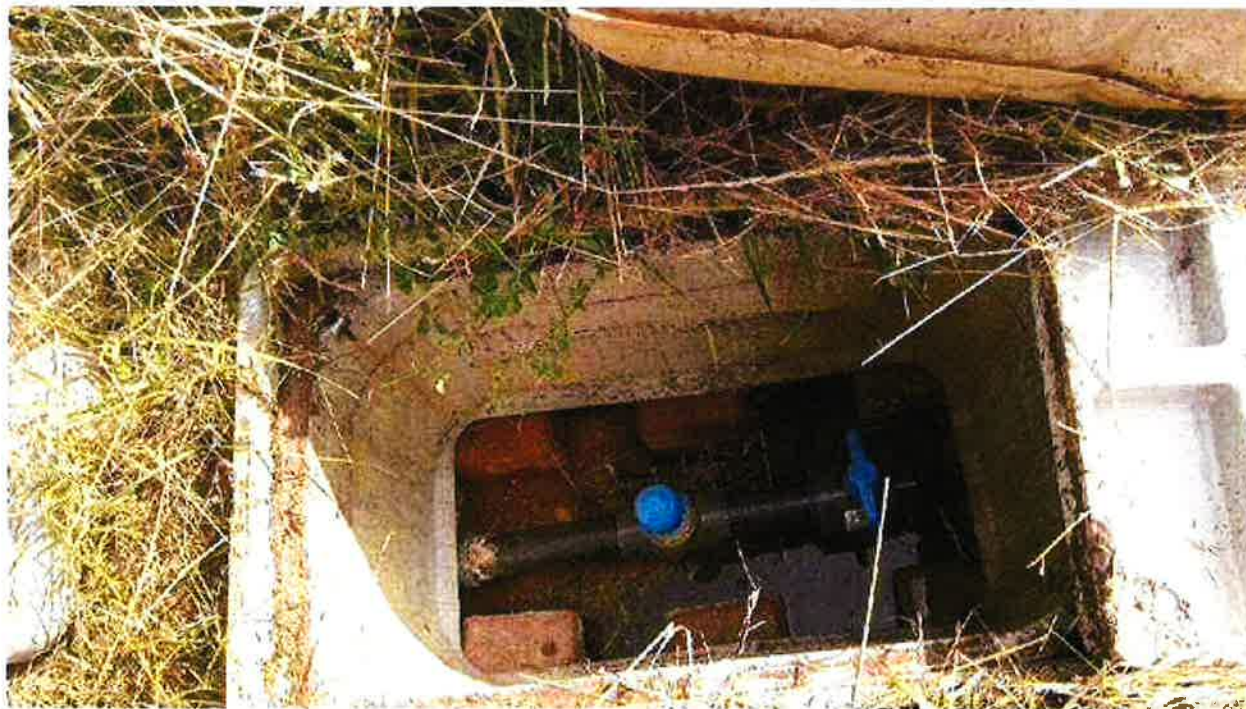
Inside Lower Ground Bed Blowoff Box
