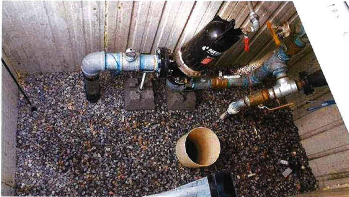
Inside Upper Ground Bed Tap/Valve Box on North Side of Pipeline
