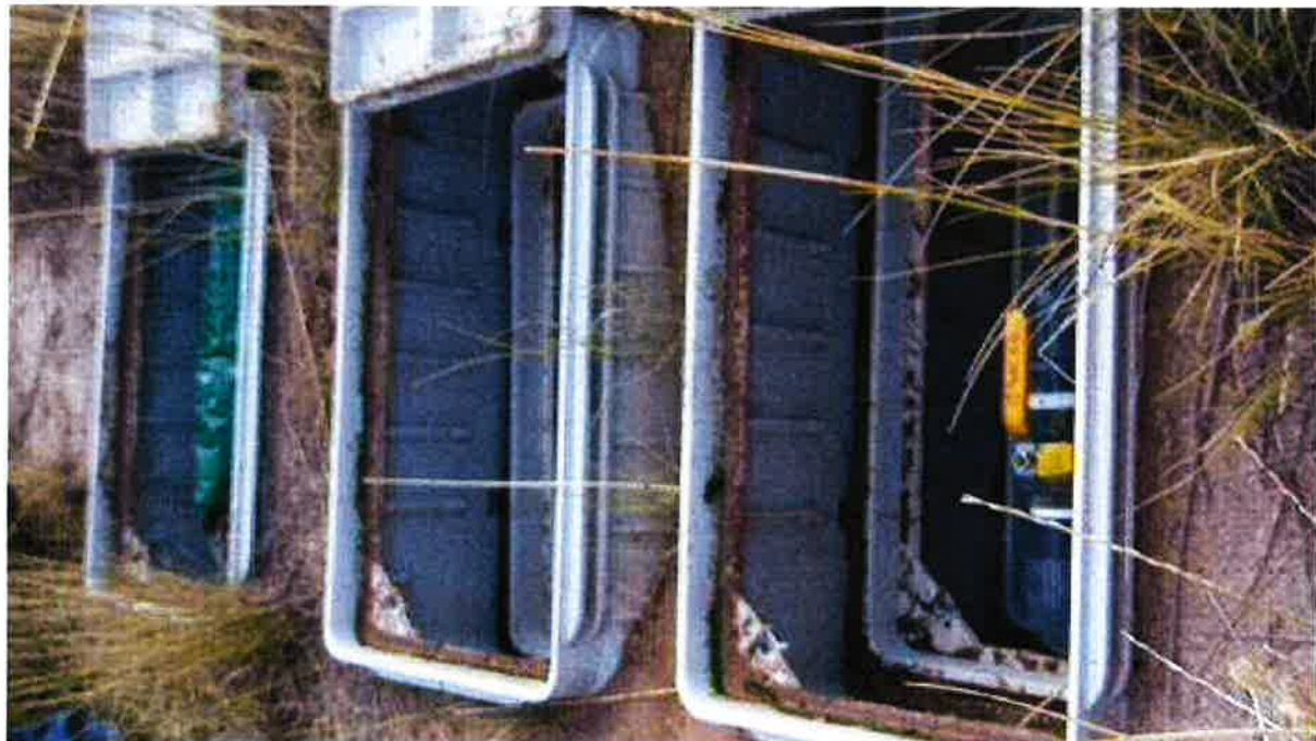
Lower Ground Bed Valve Boxes
