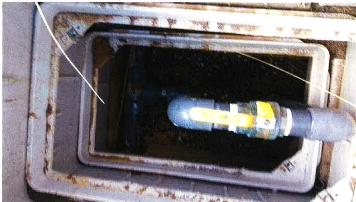
Inside Lower Ground Bed Valve Box
