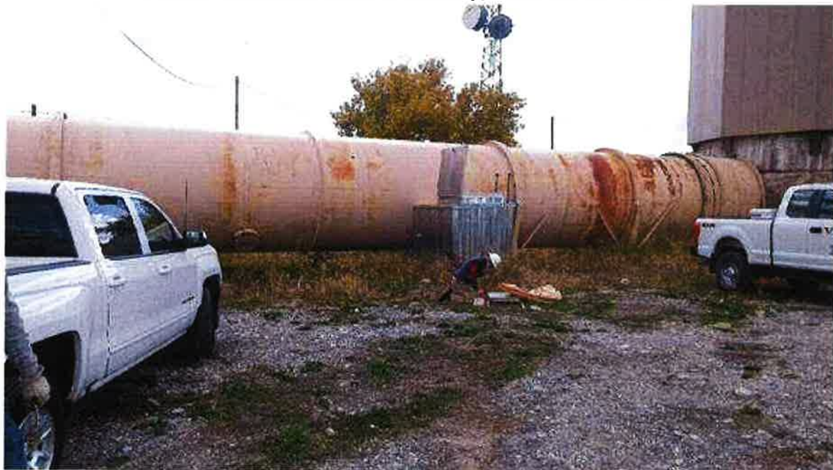
Steel Pipeline and Upper Ground Bed Above-Ground Tap/Valve Box and Buried Flow Meter Box
