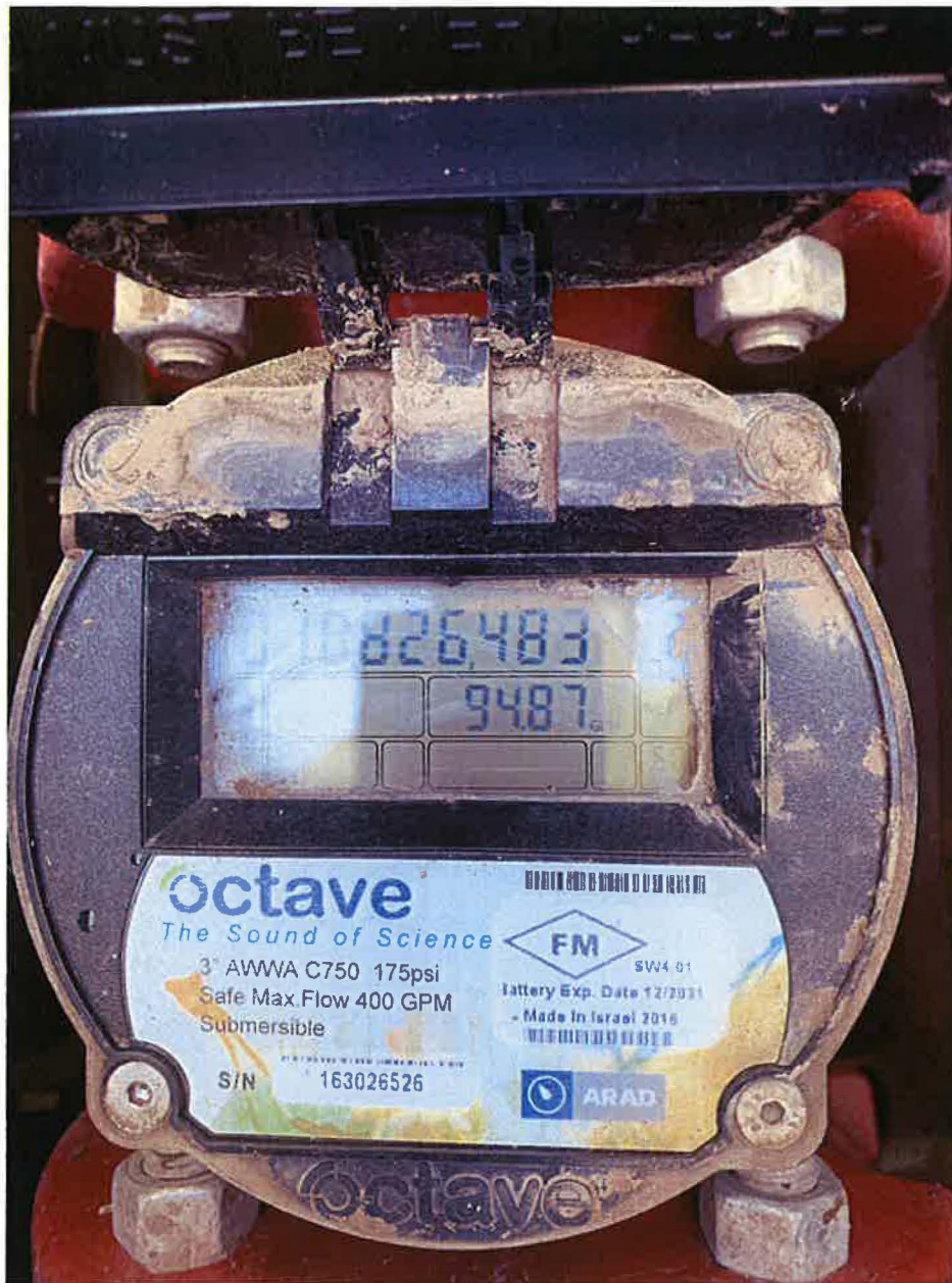
Figure 6: Northern Flow Meter.
