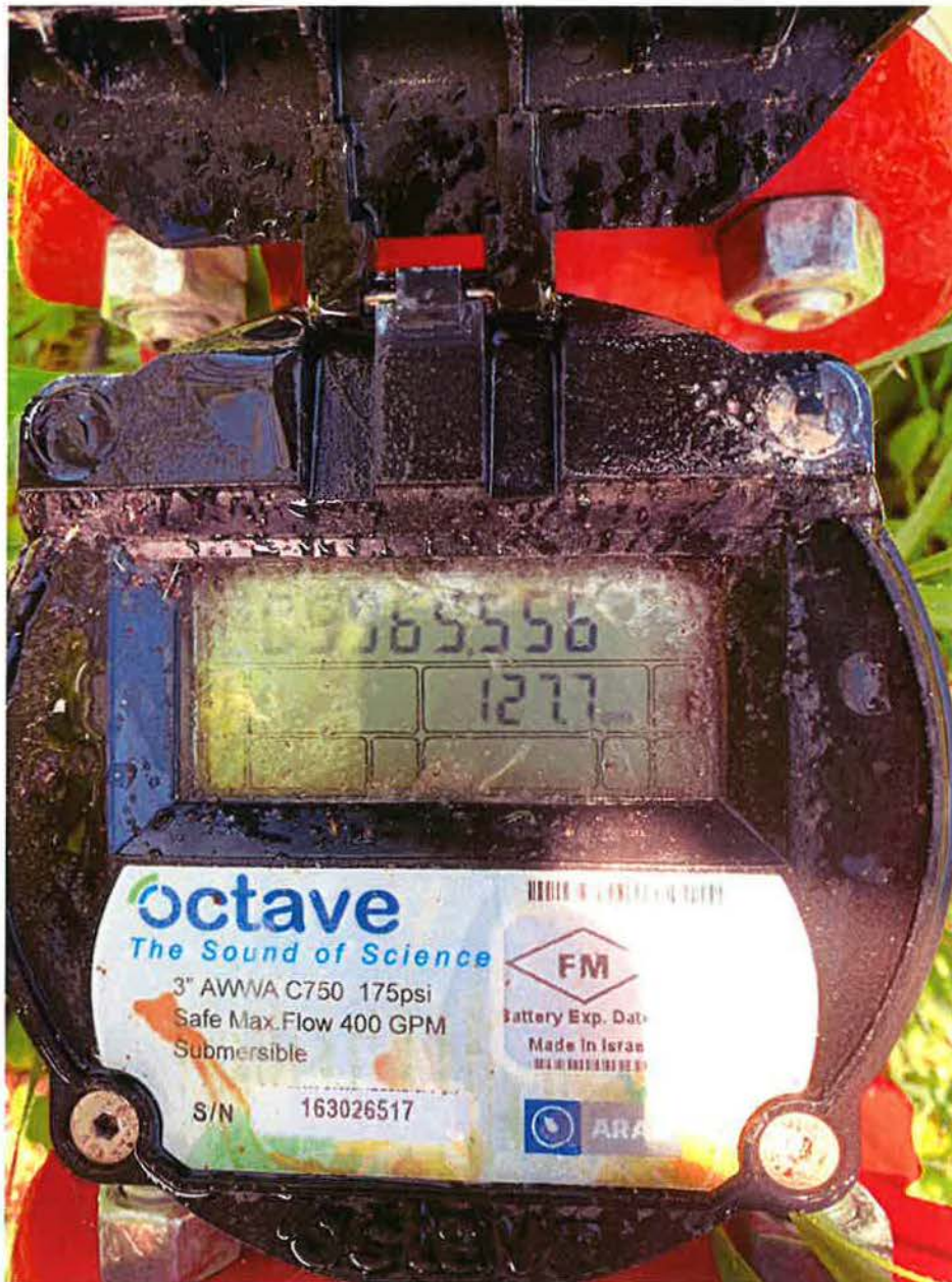
Figure 9: Southern Pump Flow Meter.
