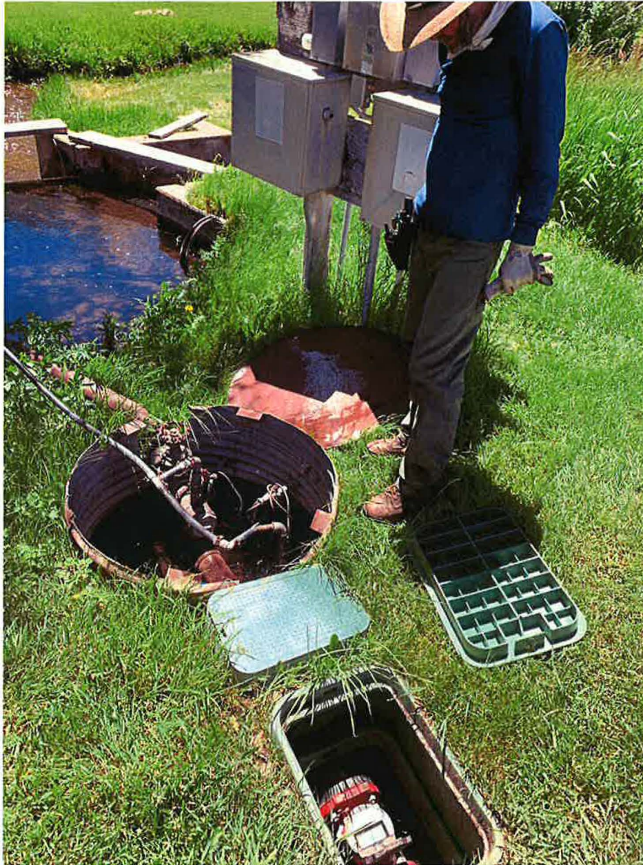
Figure 5: Seamans Creek, Verticle Sump with two Pumps, Power and Irrigation Control Panel and Northern Meter.
