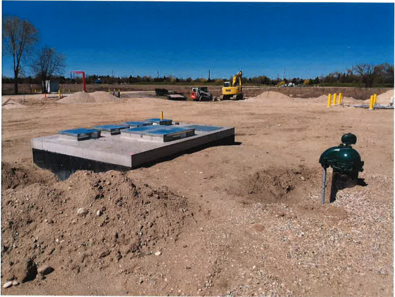
Well head and well piping/valve vault
