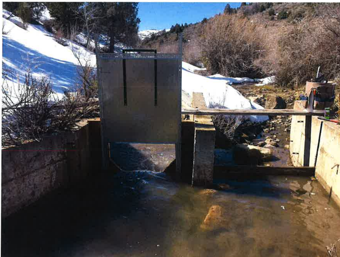
Figure 2 Example photo of slide gate.
