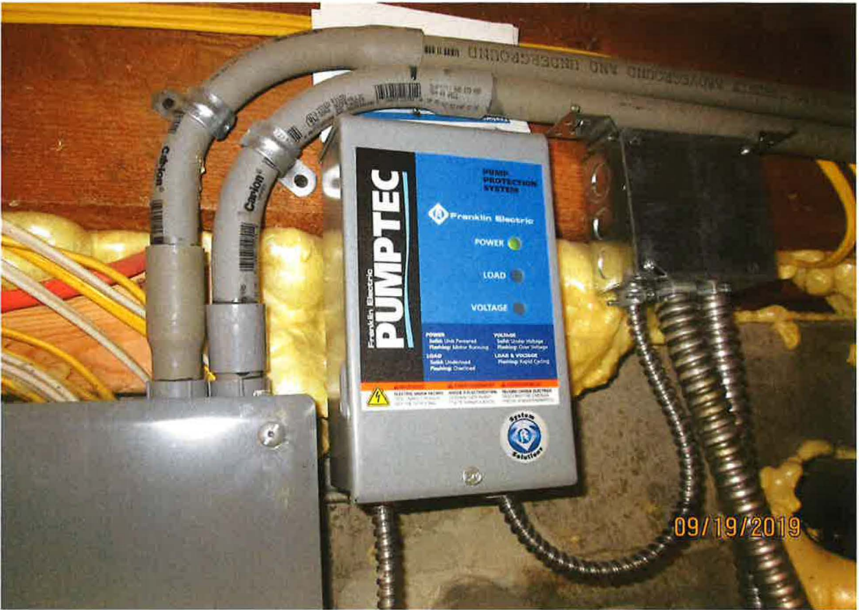
FRANKLIN PUMP ELECTRIC PANEL
