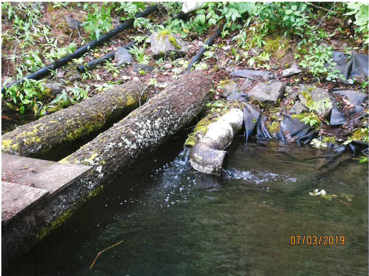
GRAVITY FED PIPE FROM CATCH BASIN AT POD
