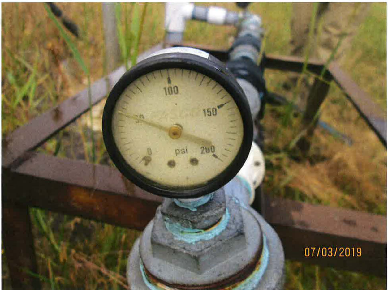
IRRIGATION SYSTEM PRESSURE GAGE
