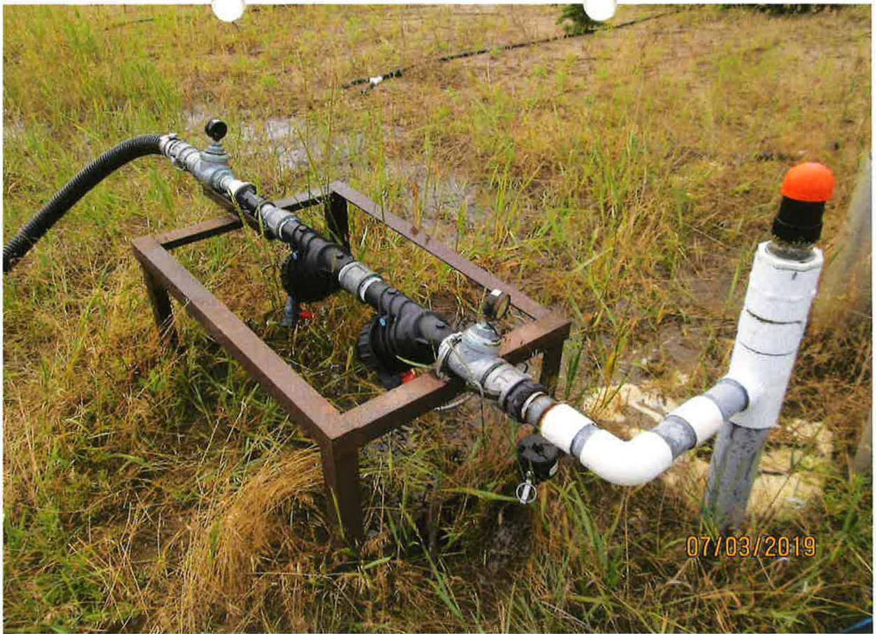
POU - IRRIGATION SYSTEM
