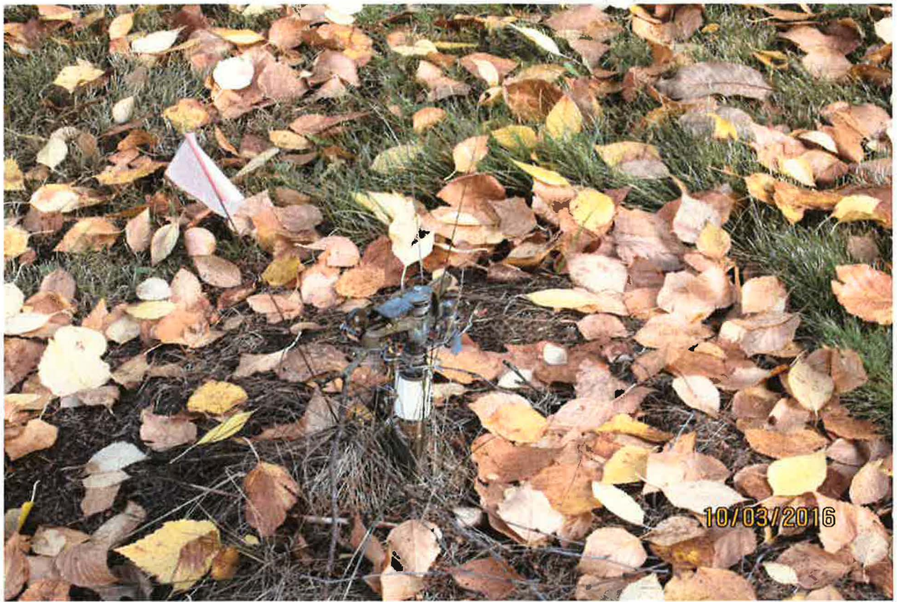
Sprinkler head in yard.
