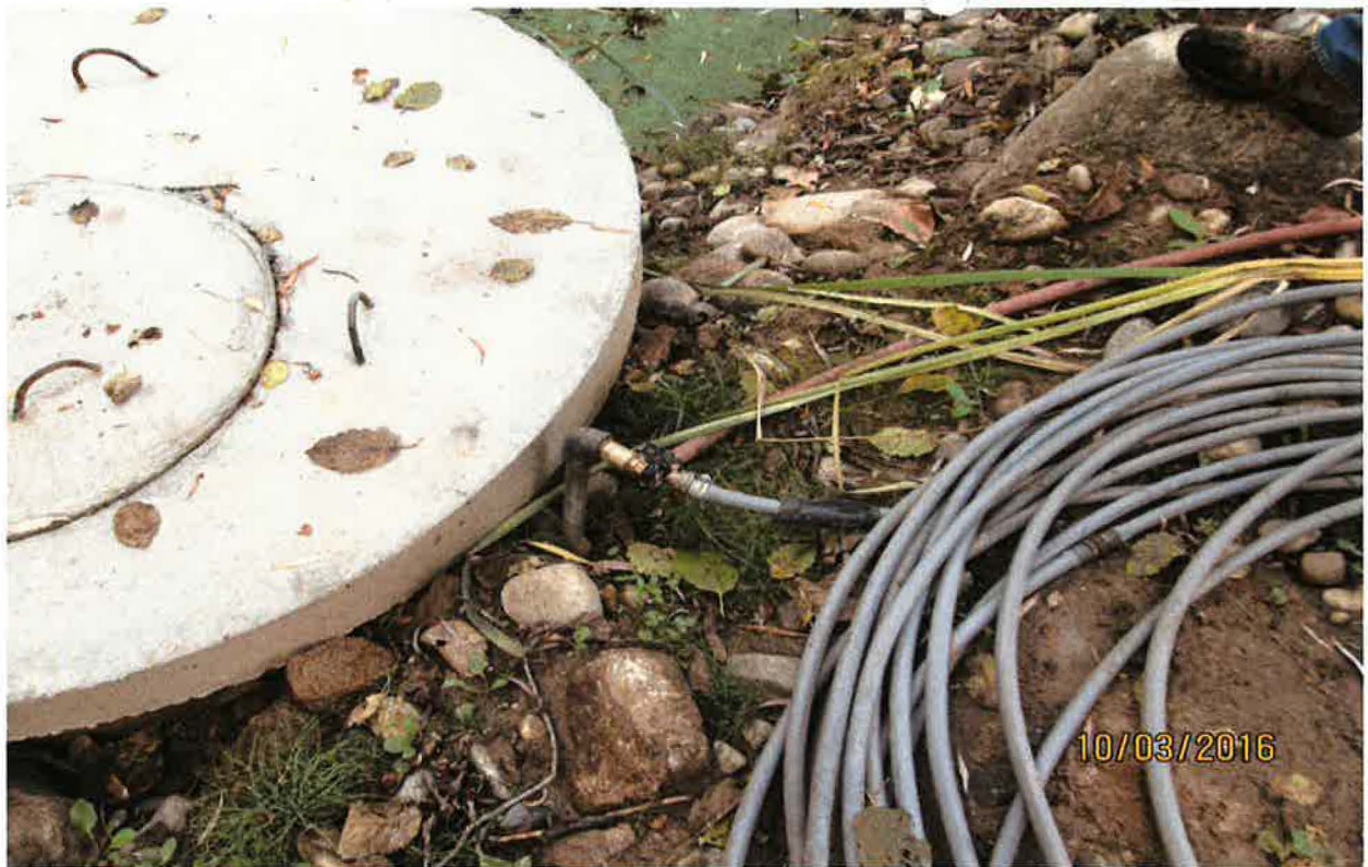
Culvert/cistern in pond with pump to use irrigation from storage from pond.
