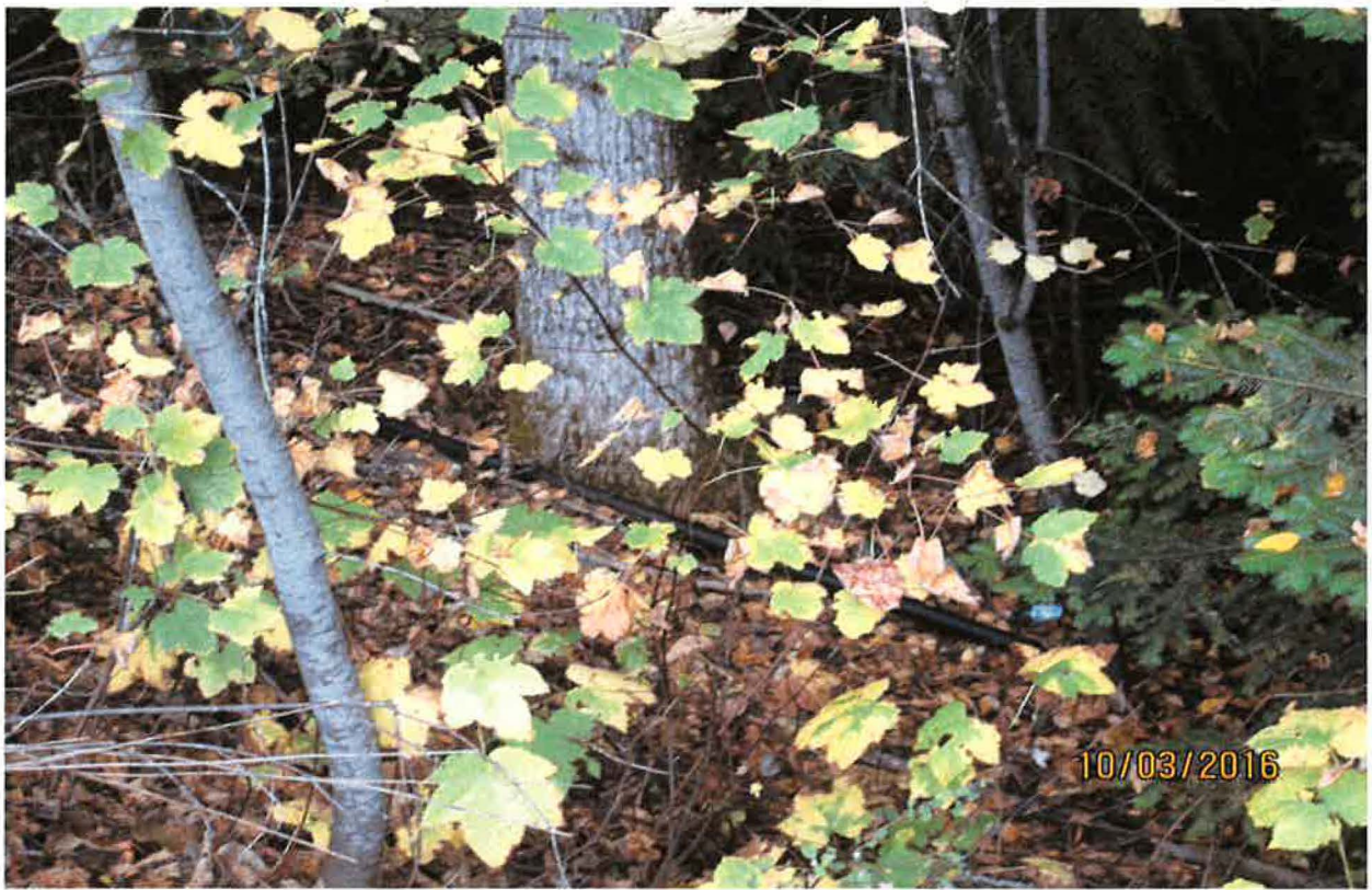
Pipe along driveway going to pond.
