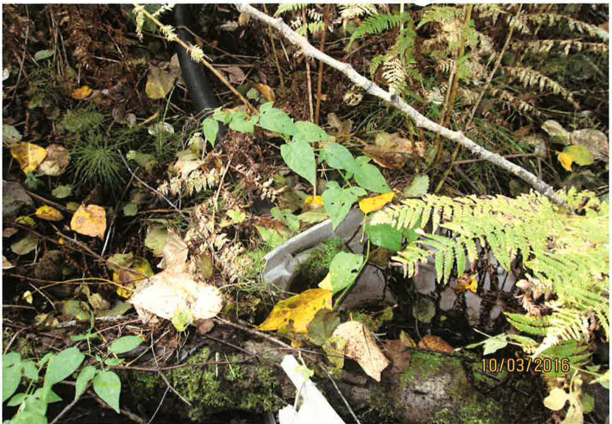
Pipe from river. Diversion to storage into pond.
