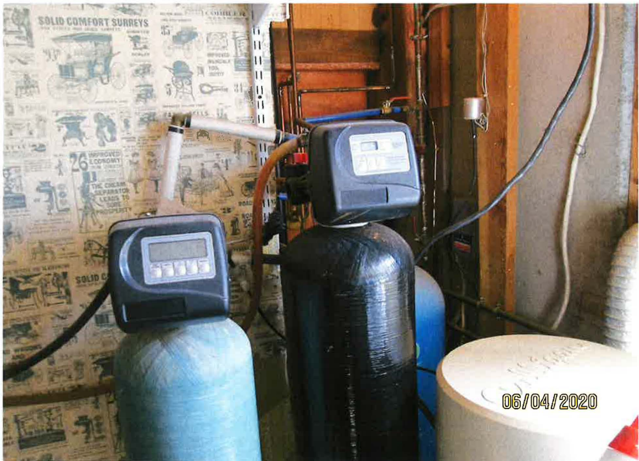
WATER SYSTEM PRESSURE TANK AND WATER FILTRATION TANKS
