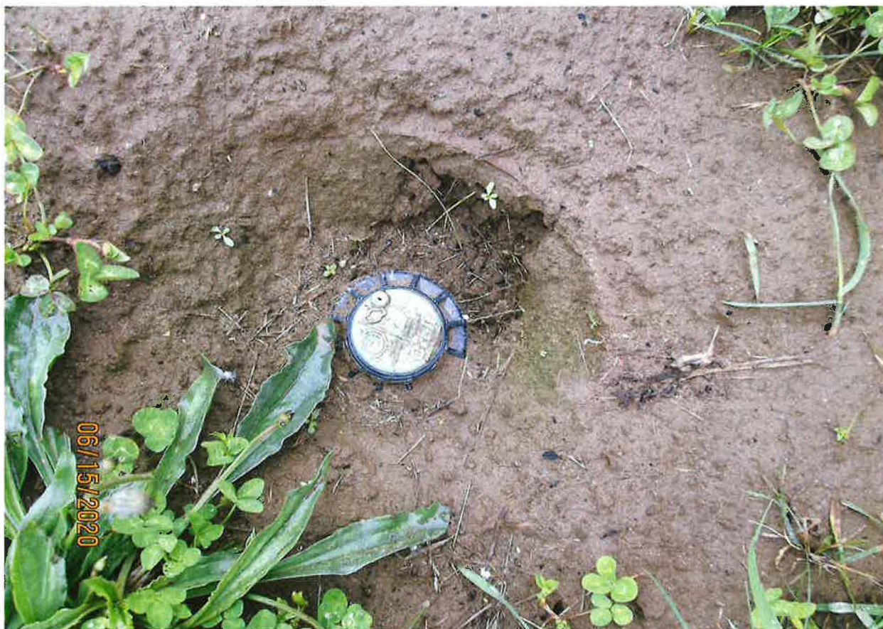
AUTOMATIC SPRINKLER SYSTEM
