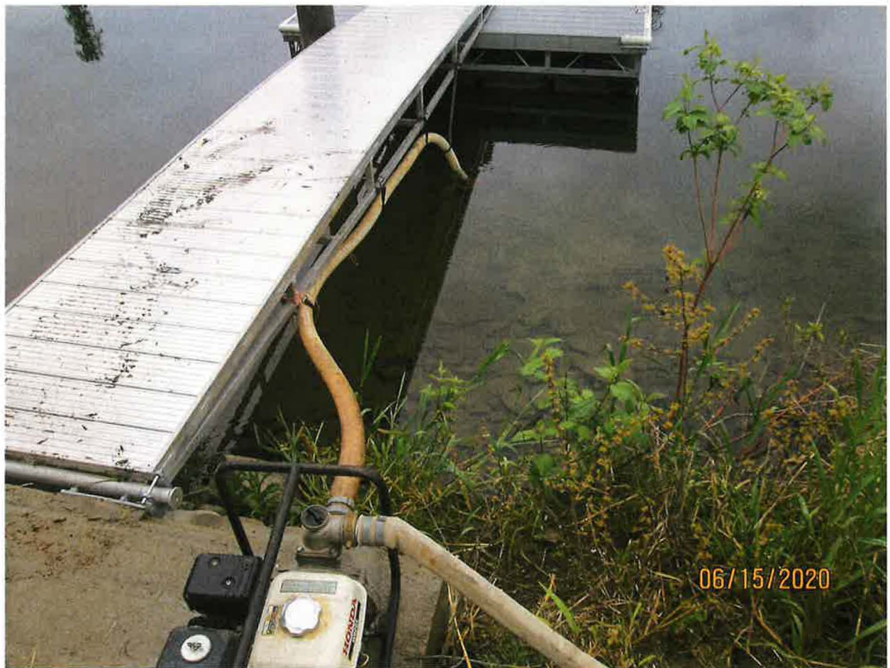
POD – GENERATOR DRIVEN PUMP
