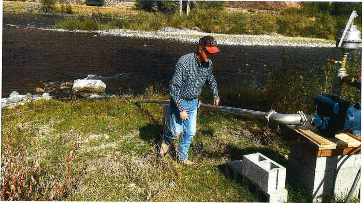
Intake in River
