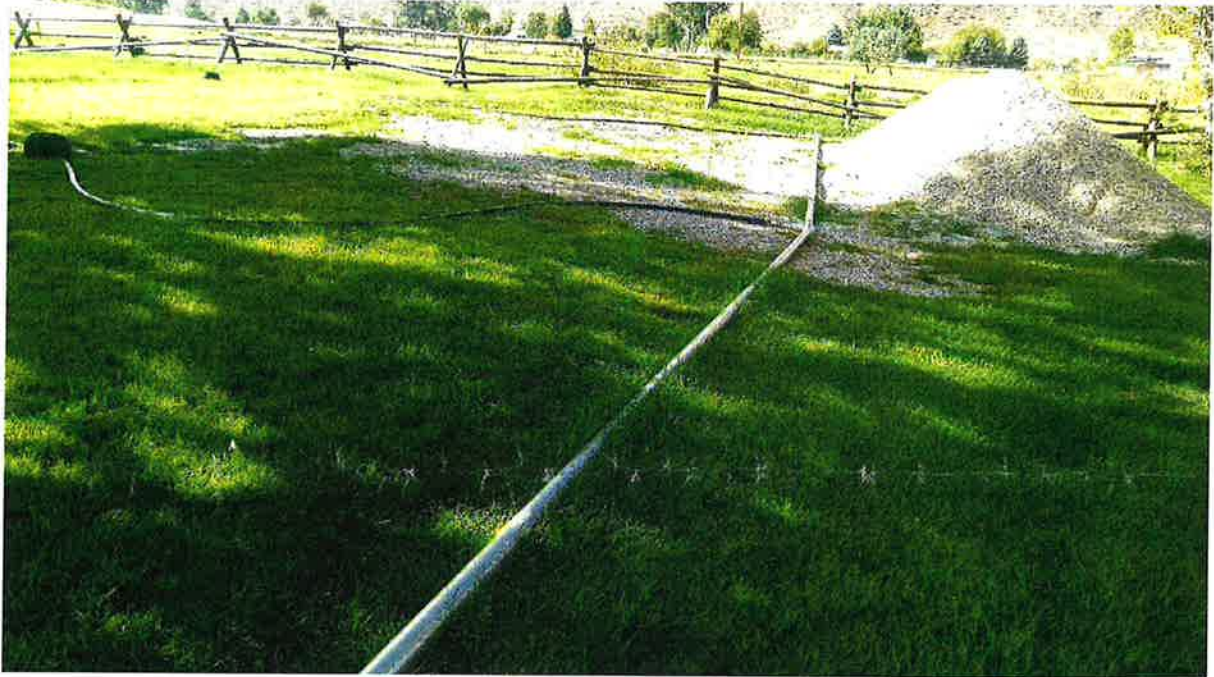
Sprinklers at South End of mainline
