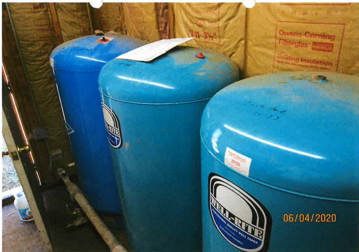
PRESSURE TANKS – LOCATED IN PUMP HOUSE
