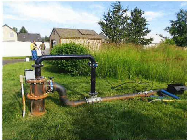
Point of Diversion, facing west towards the Pump House, which is in the southwest corner of the pond.
