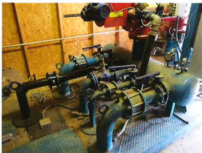
Pump system for irrigation distribution, which includes VFD & and Lag motors (outside), pony pump and recirculation motors (inside) and flushing system (black pipe) for the sand filter.
