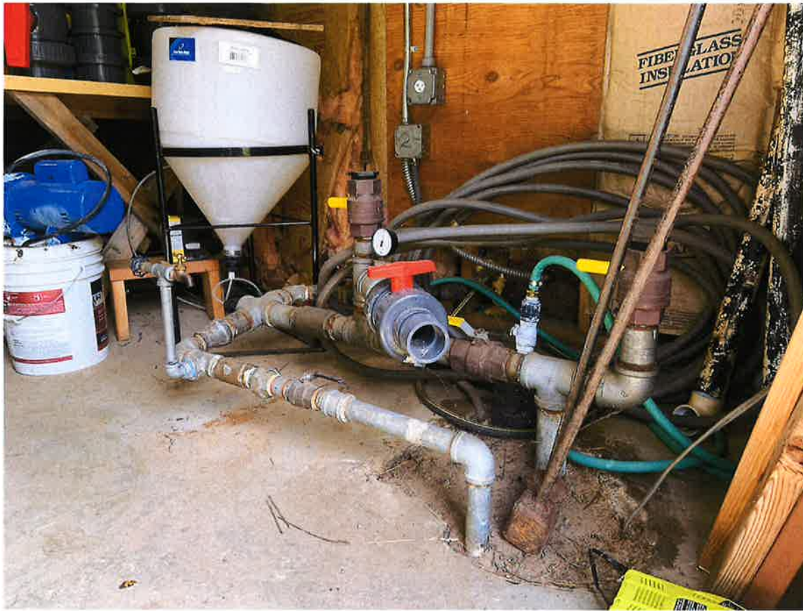
Fig. 5 – View inside pump house. Pipe in the foreground comes from Well 1, pipe in background (not seen) comes from Well 2. Larger pipe in middle is fed by both wells and goes to storage tank.
