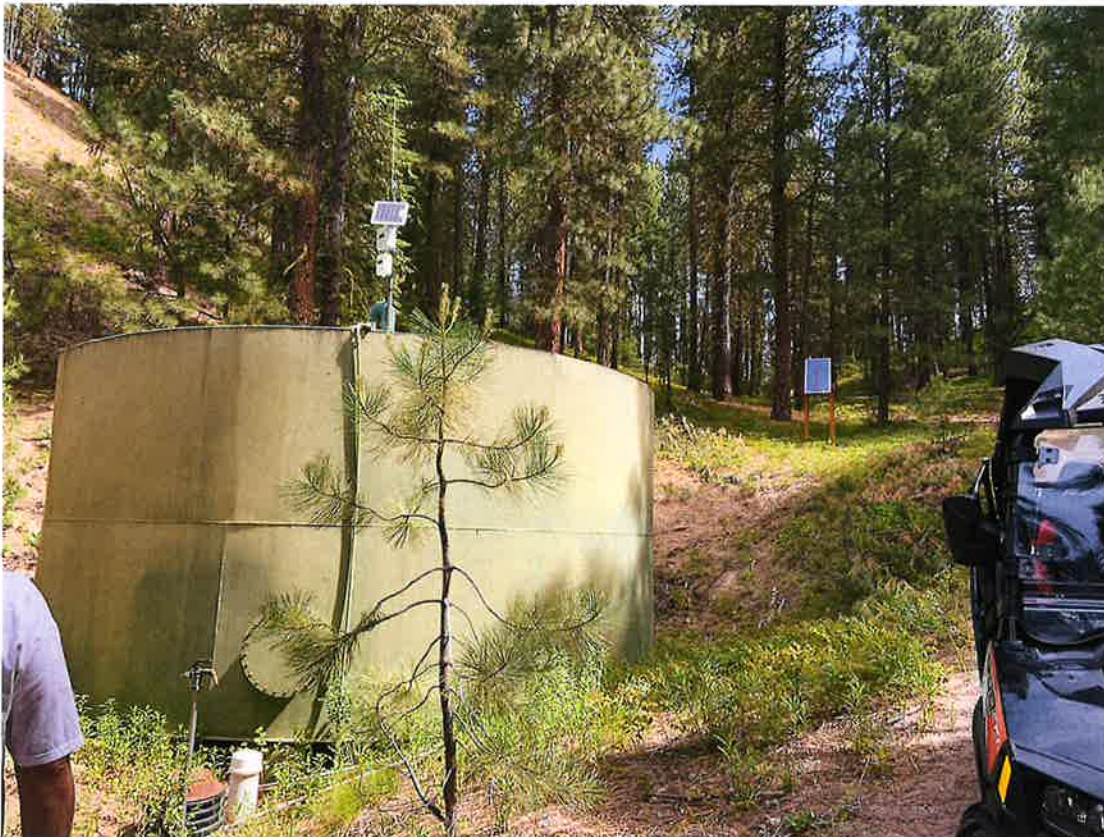
Fig. 12 – Holding tank with updated solar system in background used to power float pump switch
