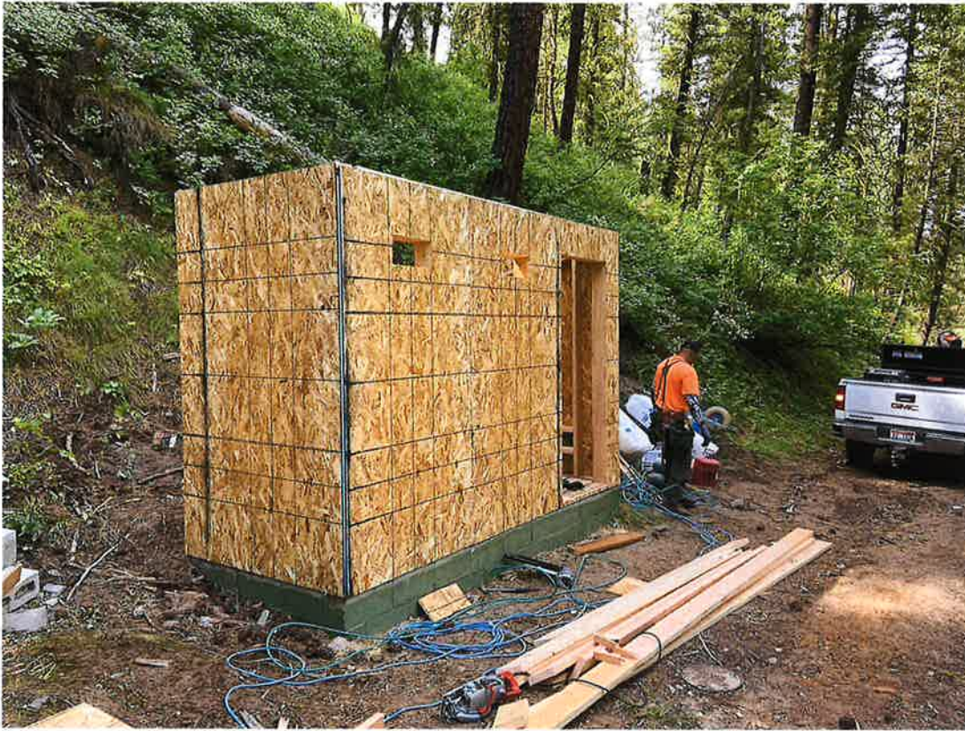
Fig. 9 – Pressure reduction system house, downhill from holding tanks. View looking east.
