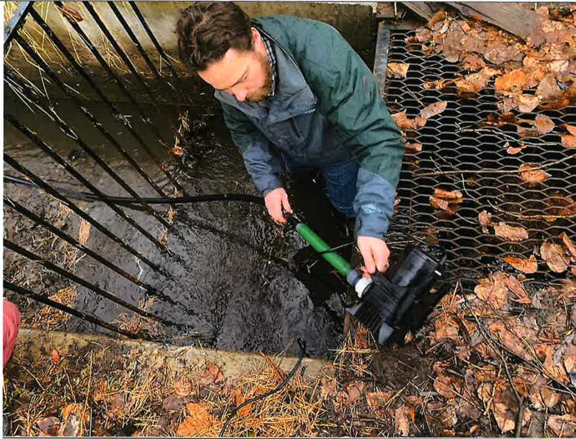
Pump used to divert water to place of use
