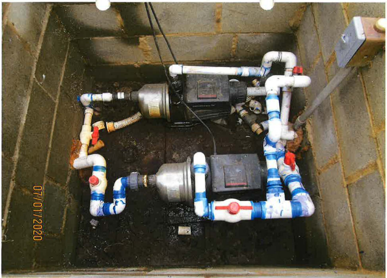
GRAVITY FED WATER FROM 2 PONDS TO PUMP HOUSE
