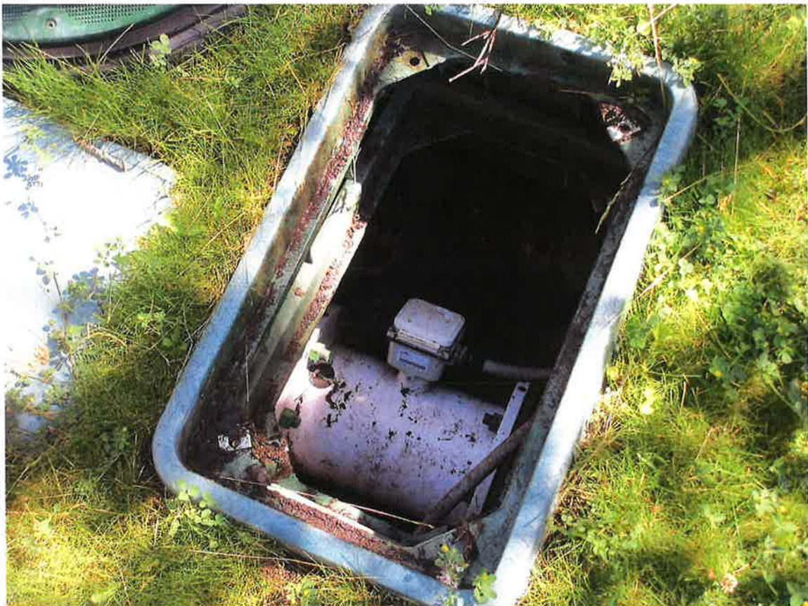
Flow meter adjacent to north well
