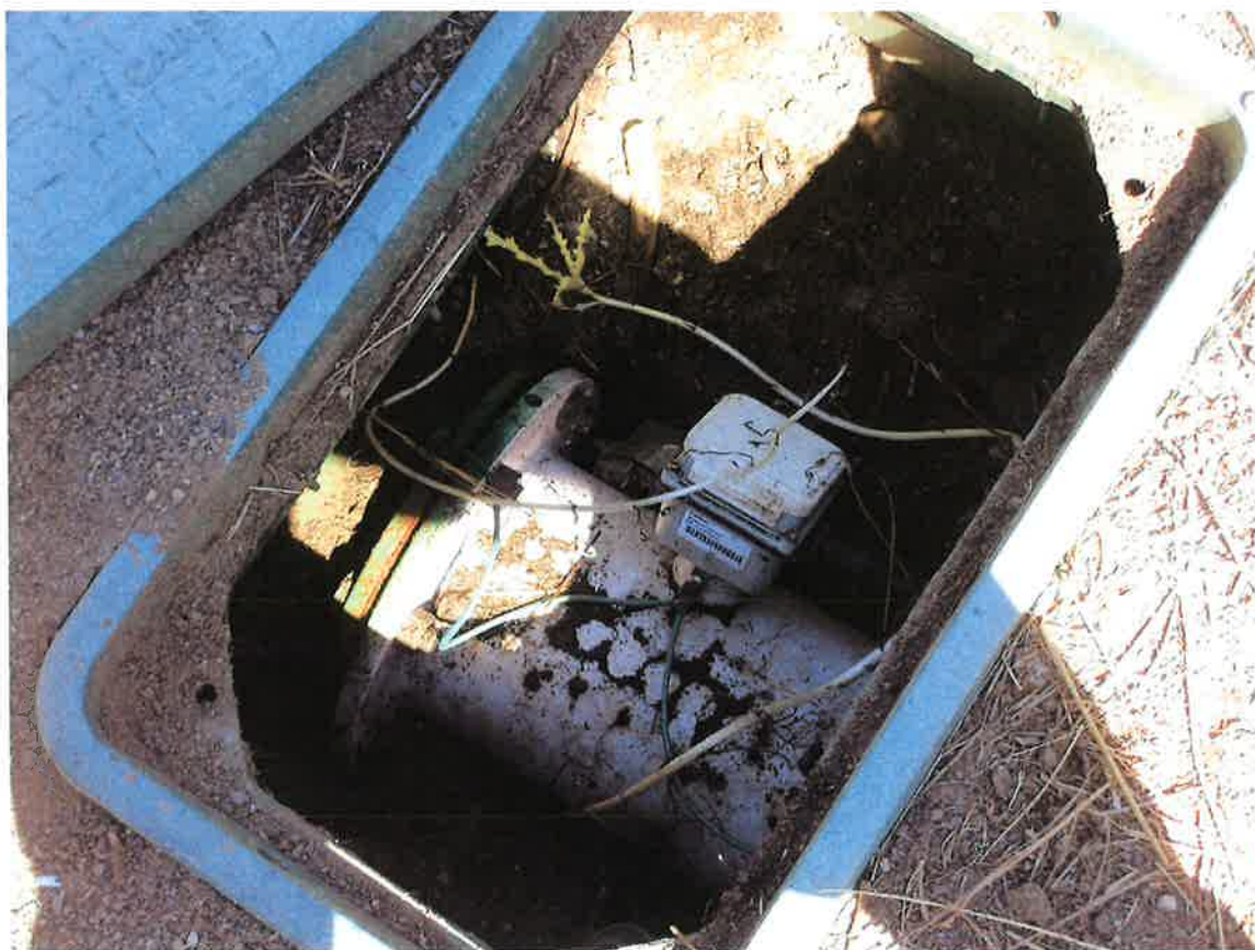
Flow meter for south well
