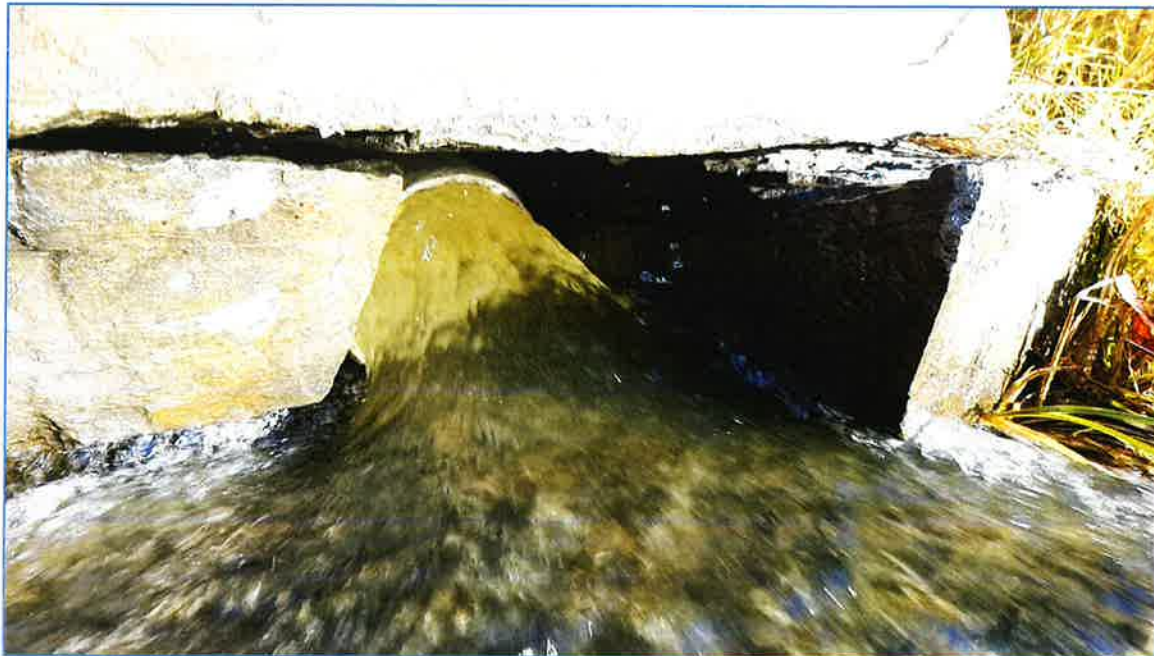
Figure 2: Pond 1 close-up of inflow into pond from 6-inch PVC pipe.
