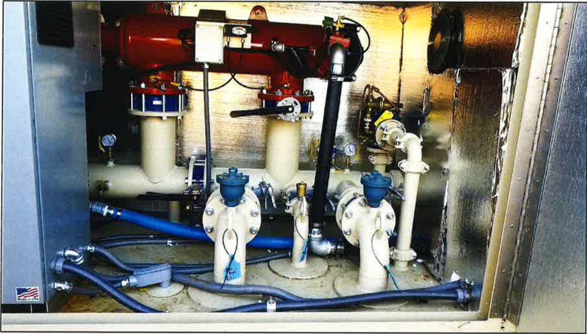
Figure 3: Mechanical piping inside pressurized pumping system.
