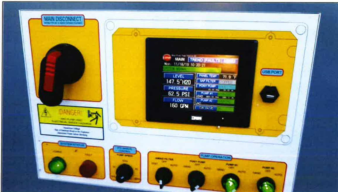
Figure 4: Pump system display shows flow which ranged from 158 to 160 gpm during exam.
