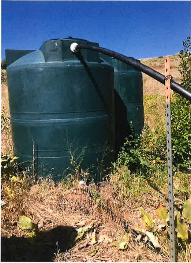
Two 825 gallon above ground storage tanks SW of POU
