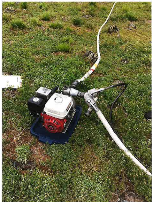
Booster pump – Honda GX160. The line in the background is the input line coming from the orchard. The 1\frac{1}{2} inch line in the fore ground goes to sprinkler #3; the black \frac{3}{4} " goes to sprinkler #2.
