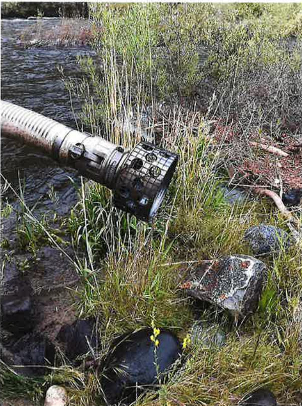
Fish screen around outside of can on suction hose.
