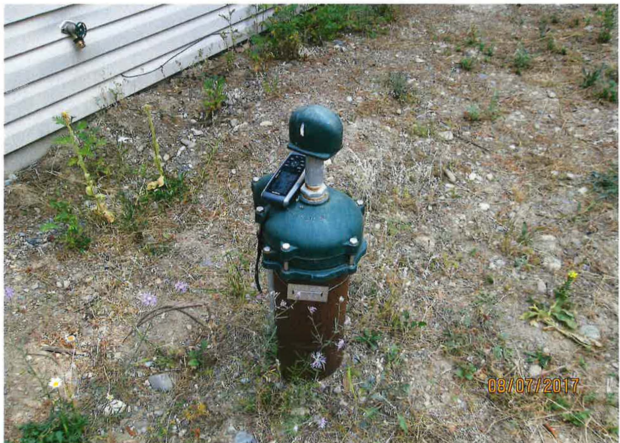
POD – WELL No. 1, A0020024
