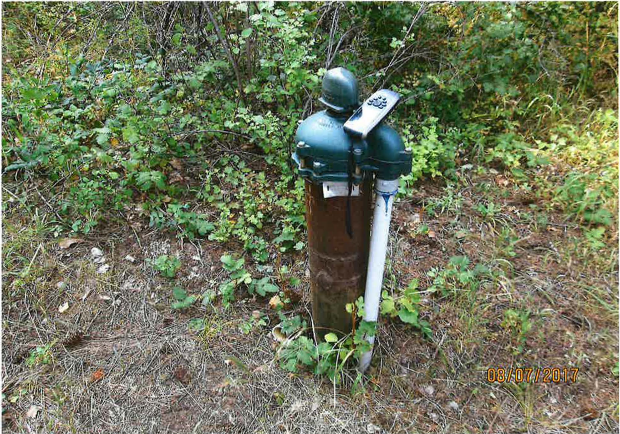
POD – WELL No. 2, A0020025
