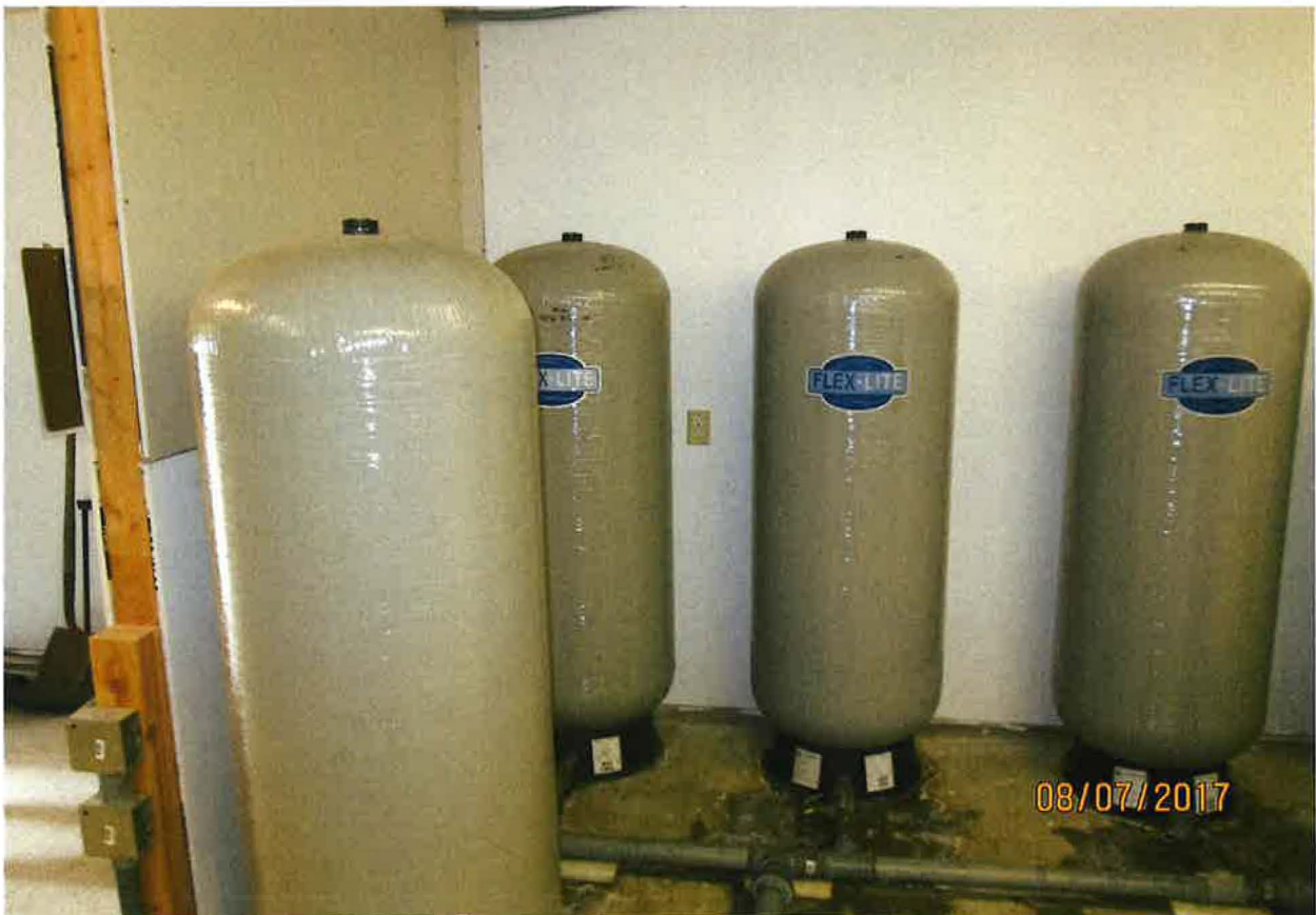
PRESSURE TANKS IN PUMP HOUSE
