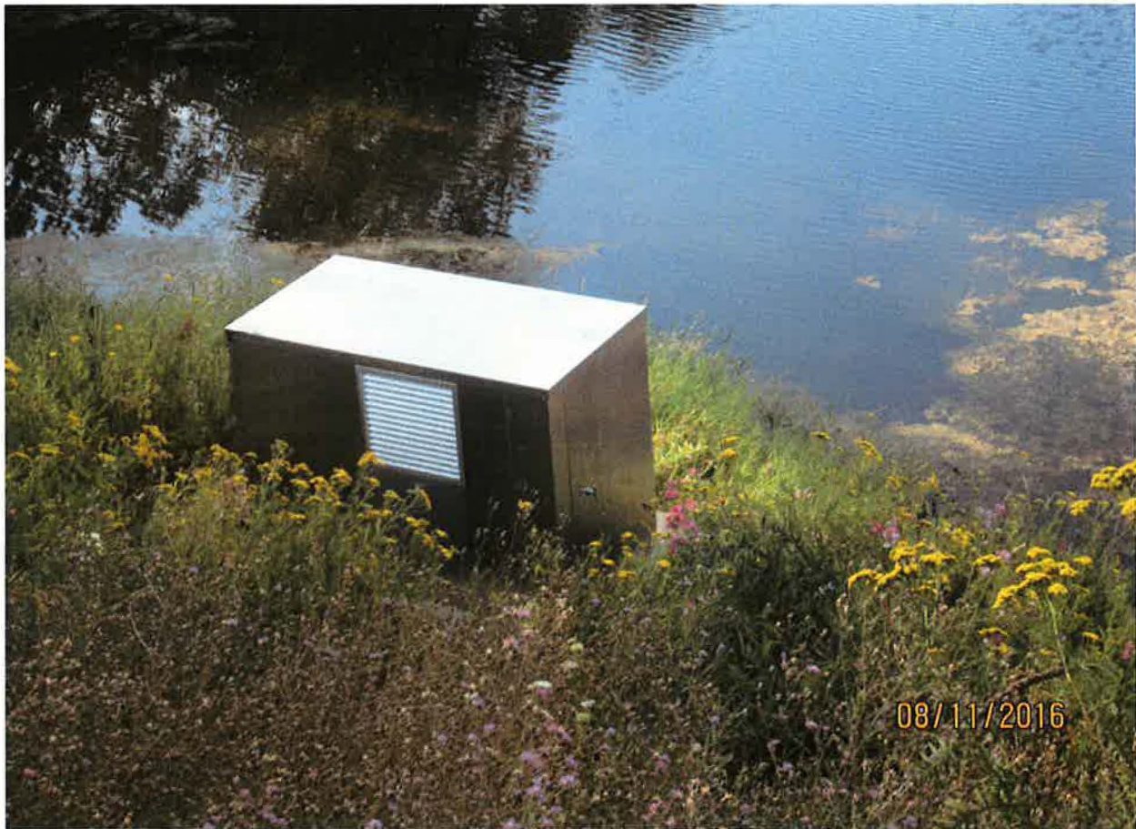
Electrical unit for pump in Chuck Slough. Director of Sandpoint's Park and Recreation Department supplied IDWR with information about system saying it is a 20 HP Hitachi motor with a Goulds #6C0C-250 250 gallon per minute pump.
