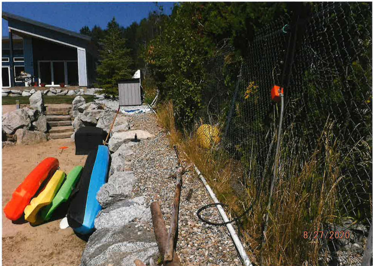
IRRIGATION SYSTEM – 1 ¼ INCH PVC PIPE ROUTED ALONG FENCE
