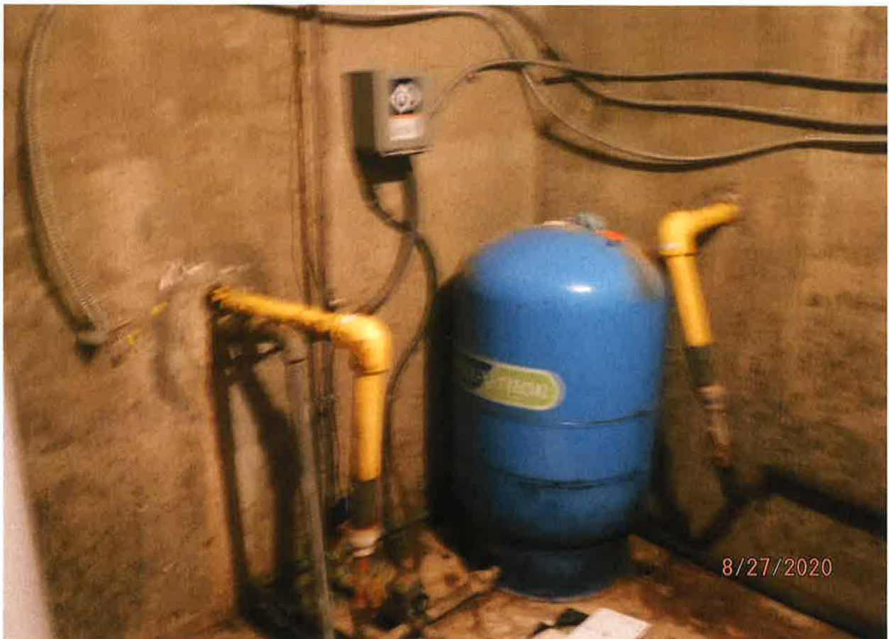
WATER SYSTEM PRESSURE TANK
