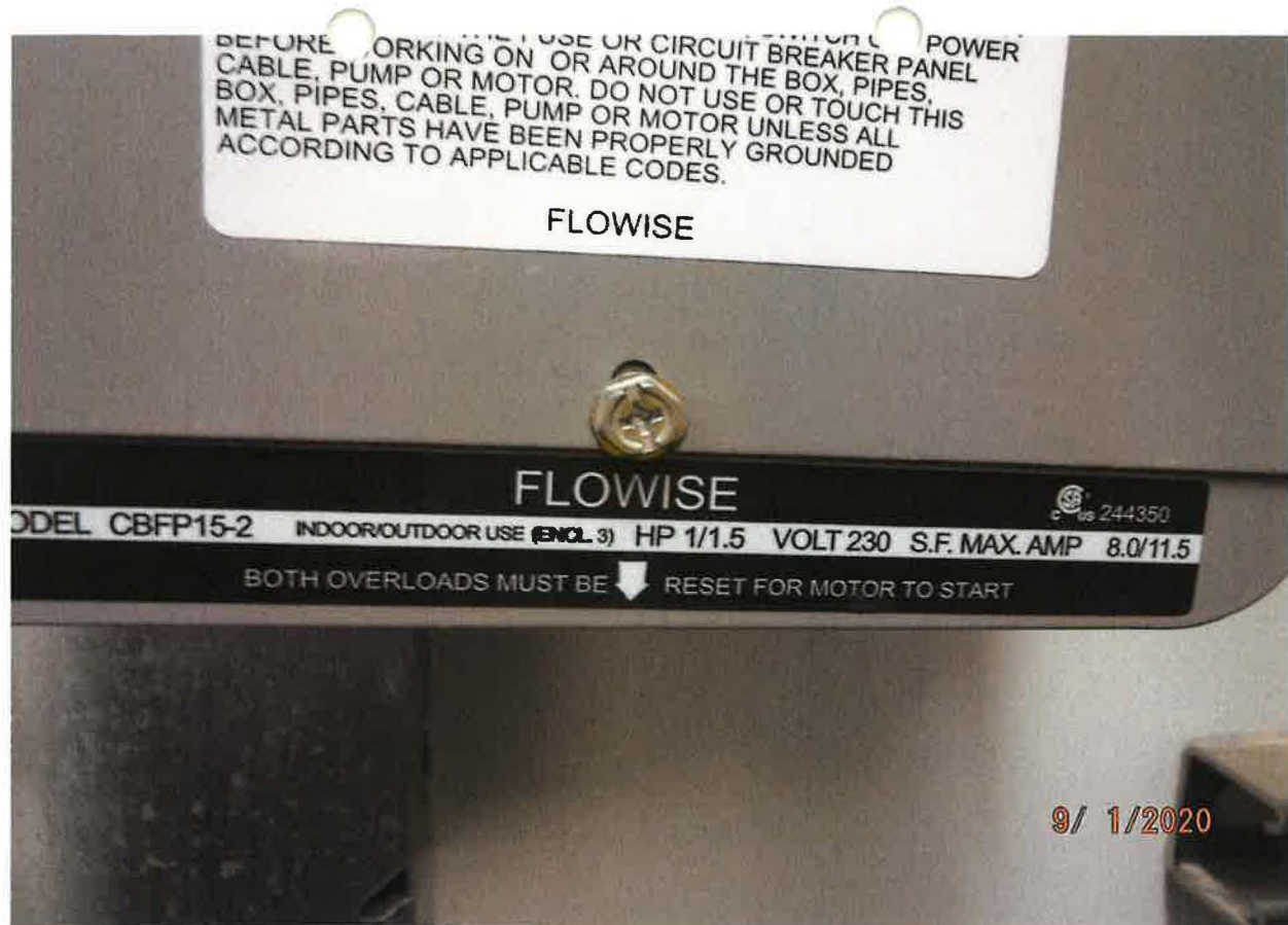
1.5 HP WELL PUMP
