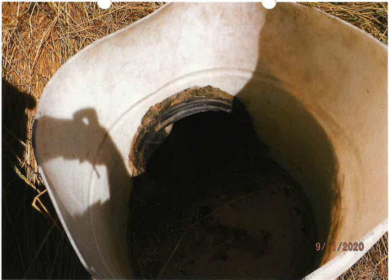
POND OVERFLOW DISCHARGE PIPE
