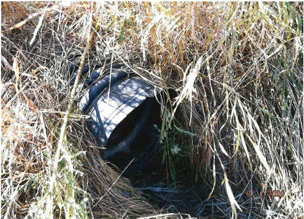
DISCHARGE PIPE EXITING POND DAM
