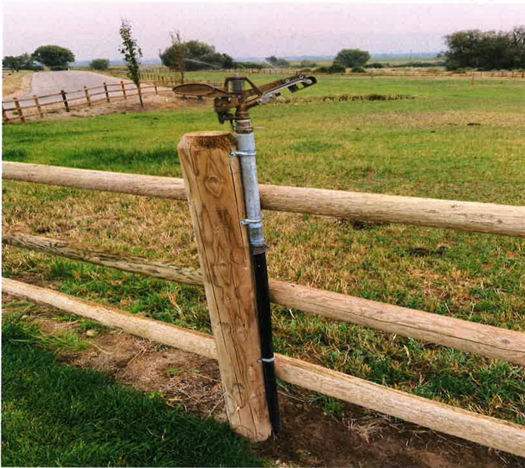
Fig. 3 – XCAD 1" Aquaburst brass impact sprinklers are along edge and down middle of pasture. Fed via 2" mainlines.
