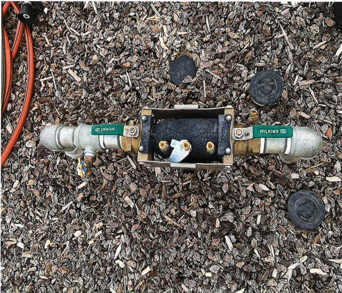
Fig. 2 – Sprinkler hookups are scattered throughout yard for attaching sprinklers/hoses.
