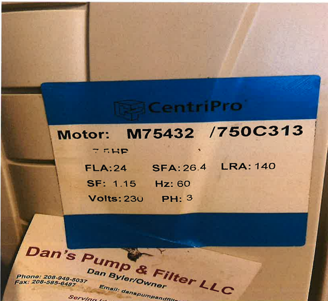
Fig. 4 – Motor control box info for system pump:
