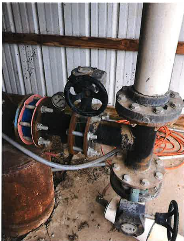
Point of Diversion (44.830064, -116.065261) 30 hp pump
