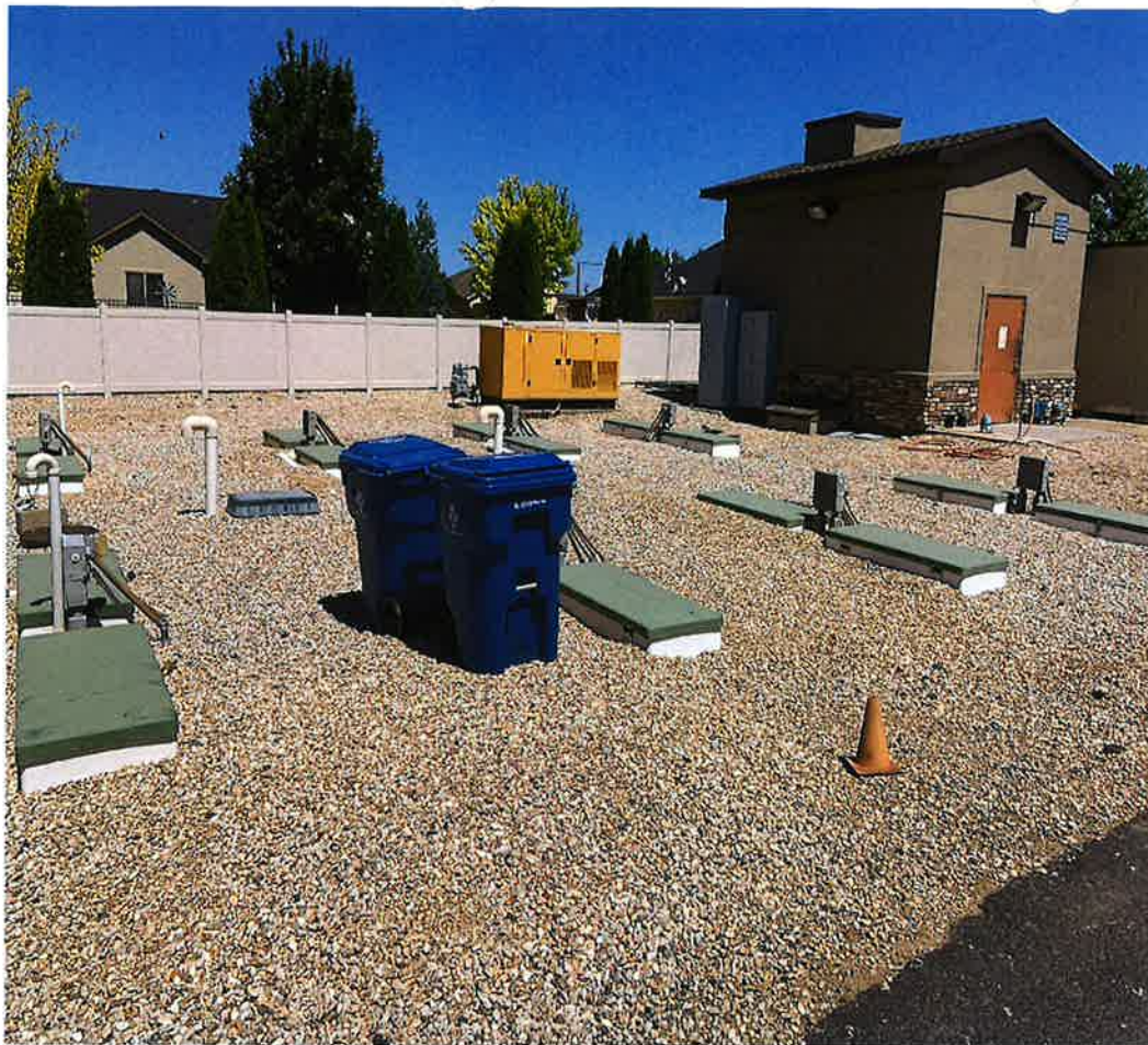
Fig. 3 – Site where wastewater/sewage from subdivision is treated. Each structure has a sub. pump to gravity system to collection pond.
