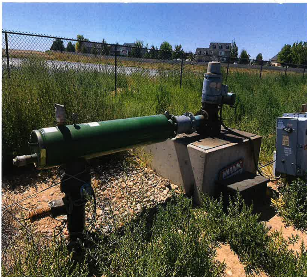
Fig. 5 – Booster pump pressurizes water from pond to sprinklers, wheel lines, etc. Collection pond in background.
