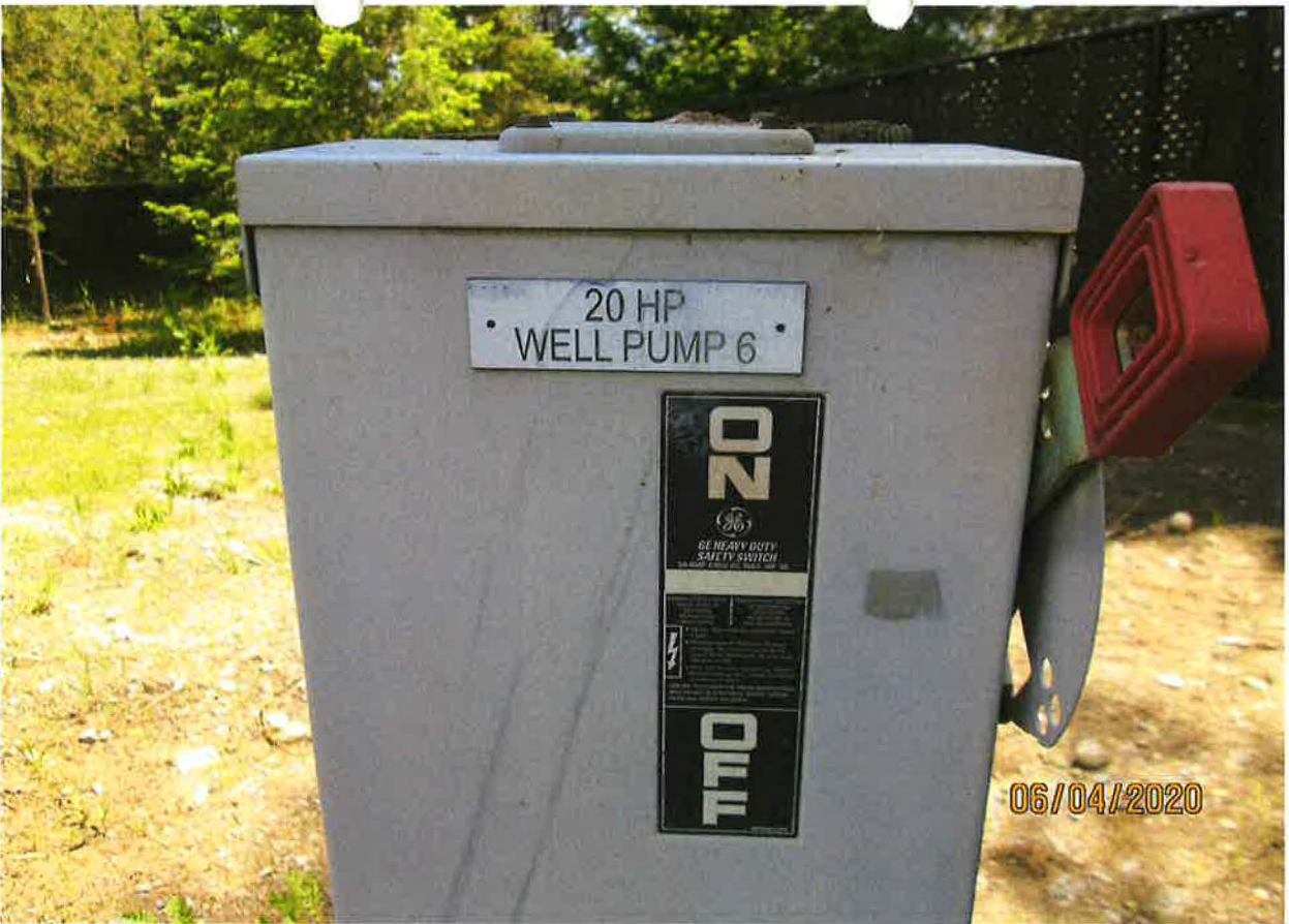
POD – WELL E0009227 – 20 HP PUMP
