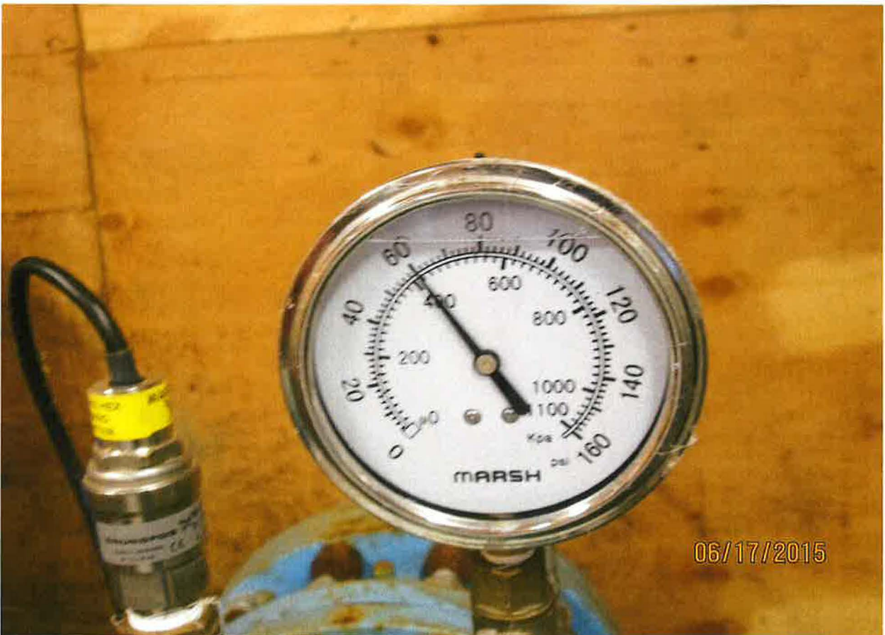
SYSTEM OPERATING AT 60 PSI
