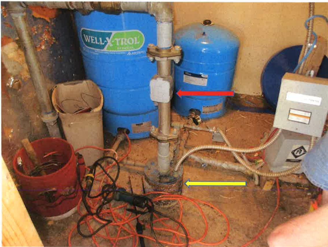
Point of Diversion (well, at yellow arrow), and flow meter (red arrow).
