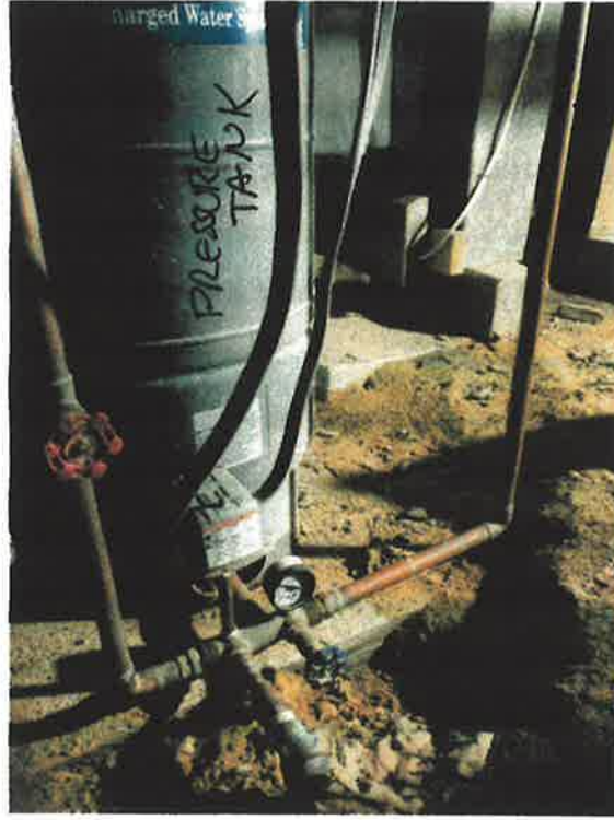
OUTGOING FROM PRESSURE TANK TO HOUSE PLUMBING - IRRIGATION
