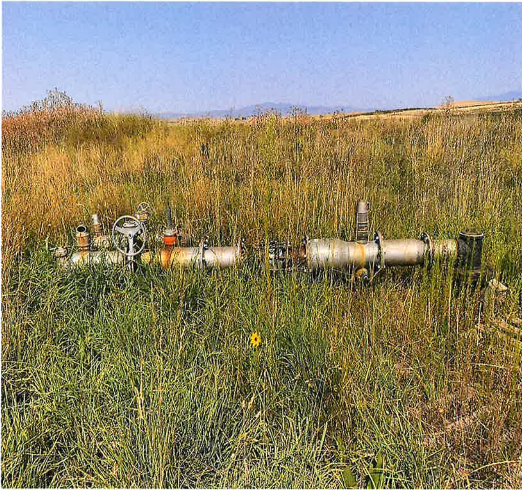
Fig. 1 – 10" diameter 418 ft deep well with 10" steel discharge line to an 8" line for pivot and 6" line to solid set sprinkler lines.
