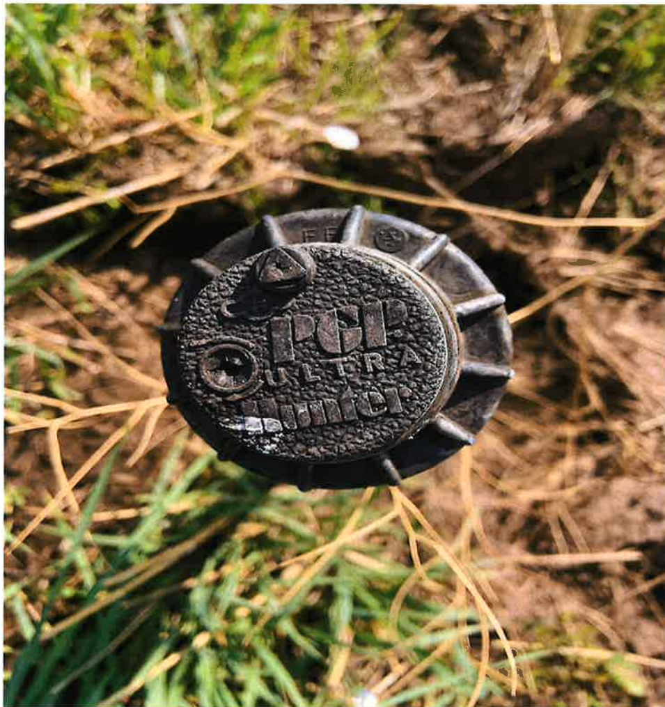
Fig. 7 – Close up view of Hunter PGP Ultra solid set sprinkler
