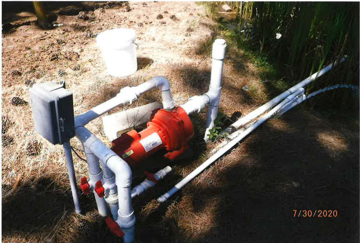
2 HP PUMP FROM 24HR CONTAINMENT POND SERVICING IRRIGATION AND STOCKWATER POU's
