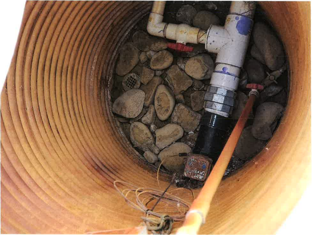
Above: Inside view of the meter and the pipe connected to the well head
