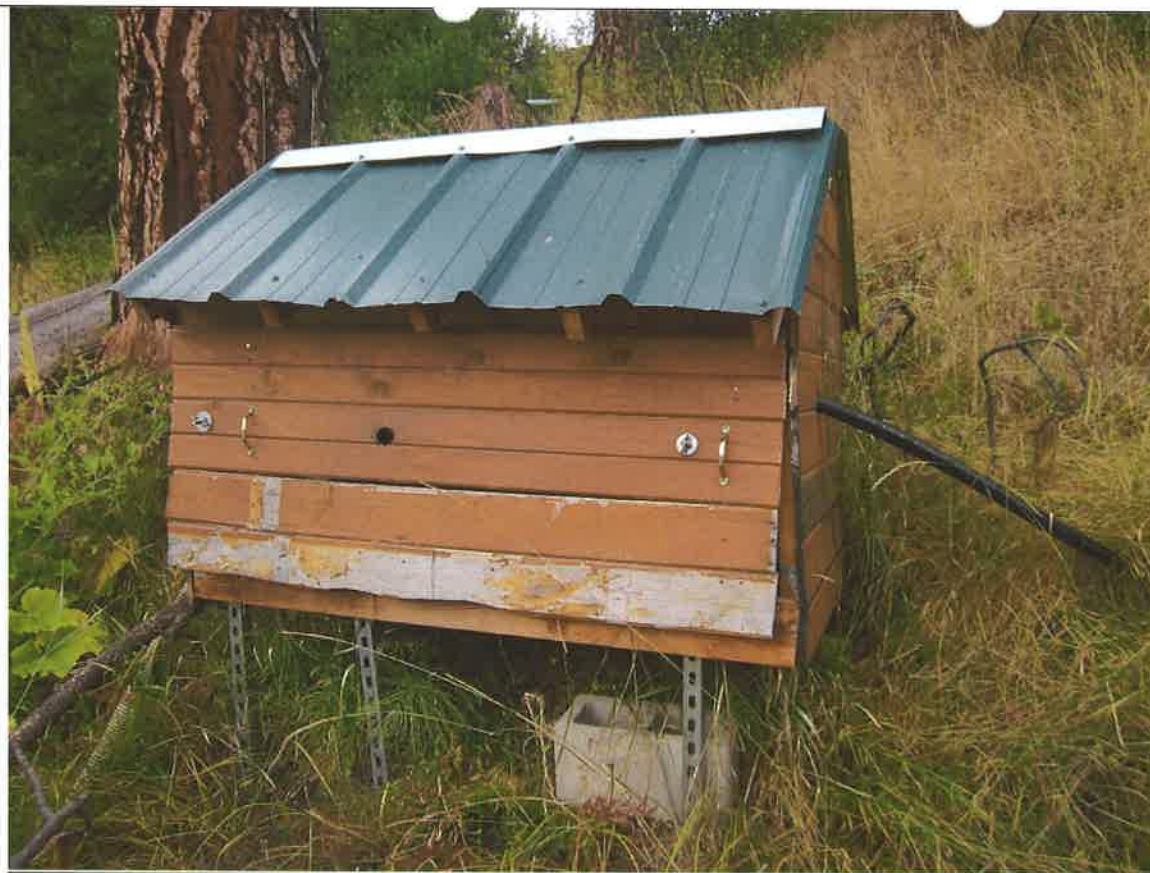
Figure 1. Pump house with 2" discharg line to irrigate lawn.
