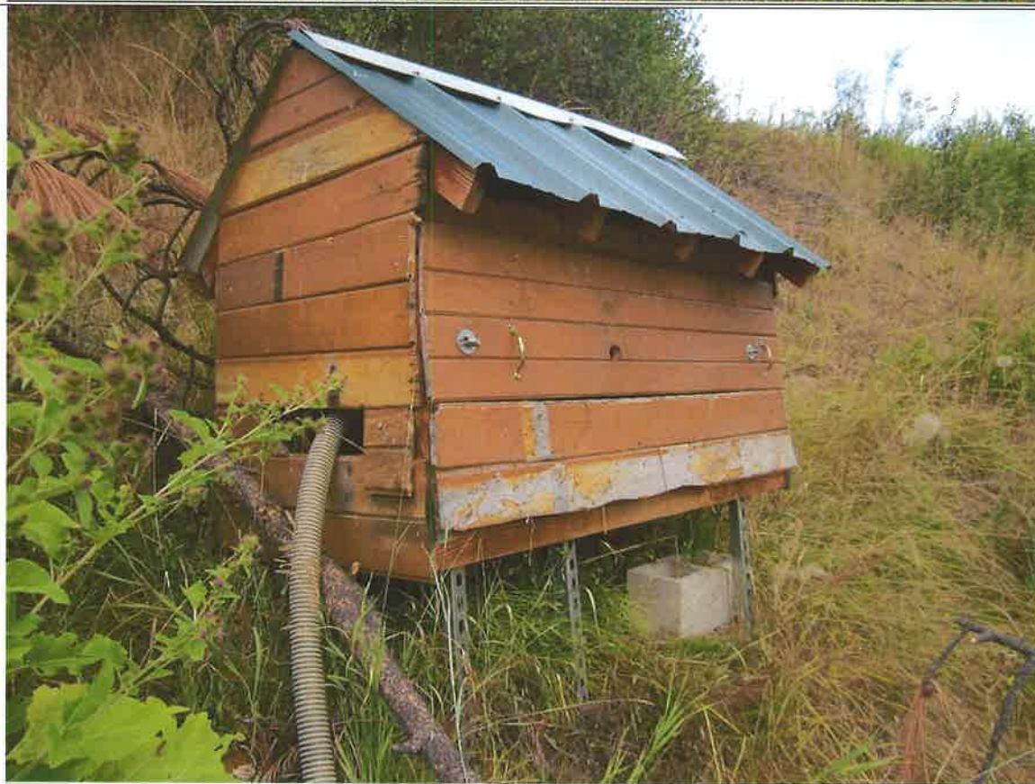
Figure 2. Pump house with 2" suction hose with approximately 12 feet of lift from Middle Fork Payette River.
