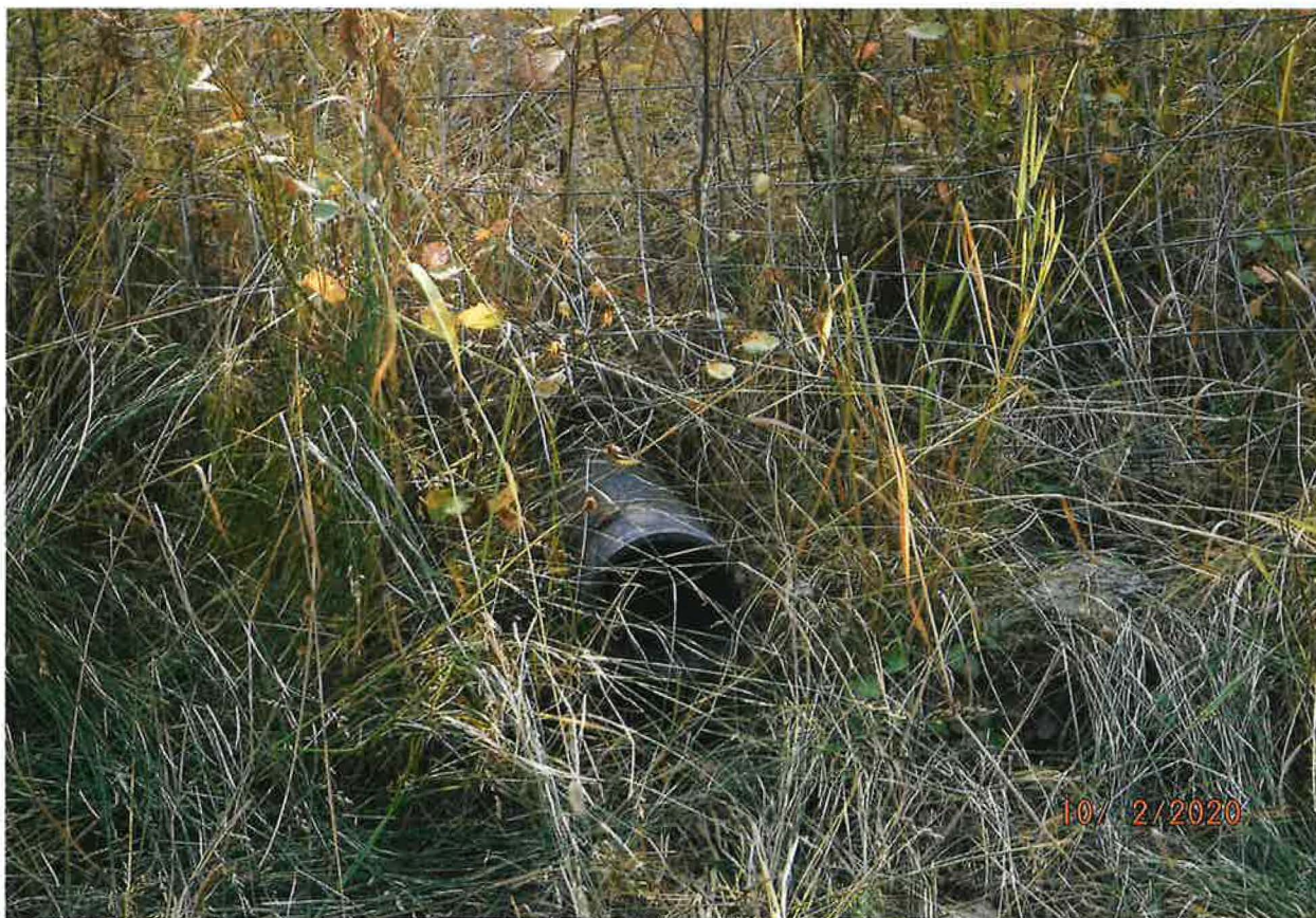
POND OVERFLOW DISCHARGE PIPE INTAKE
