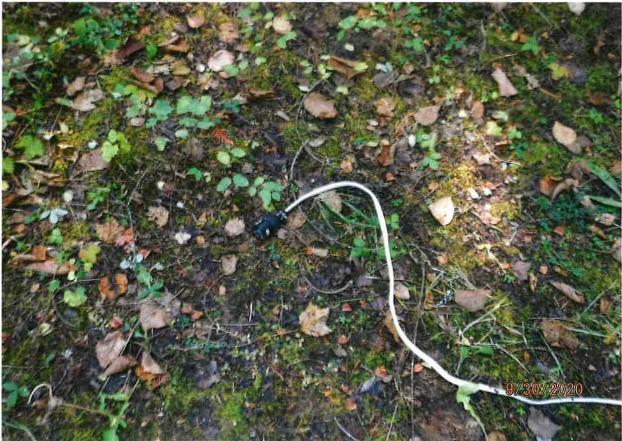
POWER CORD FOR WATER TRANSFER PUMP LOCATED AT POND
