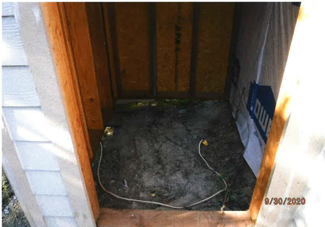
STORAGE LOCATION FOR PORTABLE WATER PUMP AND ELECTRICAL STUB
