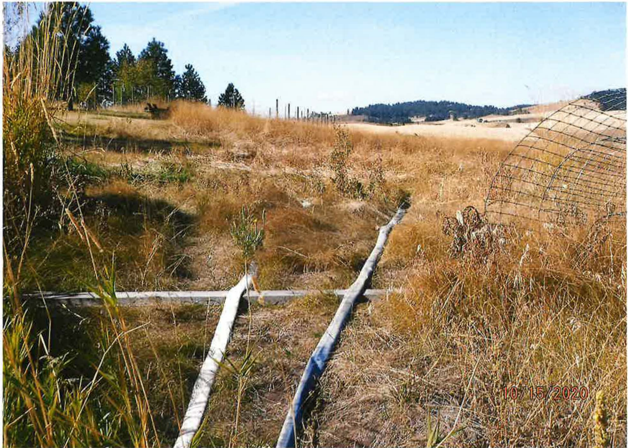
FIRE HOSE PATH FROM POND 1 TO IRRIGATION FROM STORAGE POU (IN BACKGROUND)
