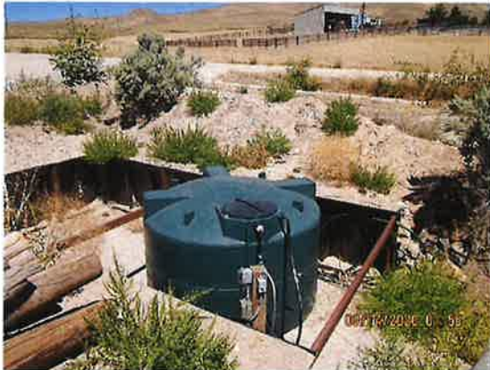
Storage tank. Sandypoint Lane in background.
