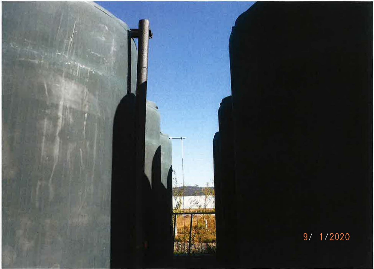
6EA 5,000 GAL STORAGE TANKS
