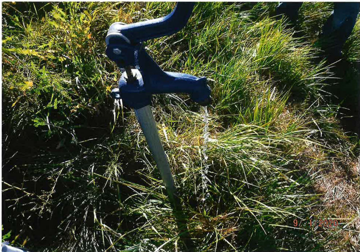
FROST FREE HYDRANT PIPED DIRECTLY OFF WELL MAIN LINE
